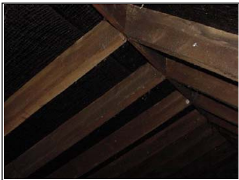
Ridge Board and common rafters (the ones which form the pitch of the roof) showing minimal signs of movement.
