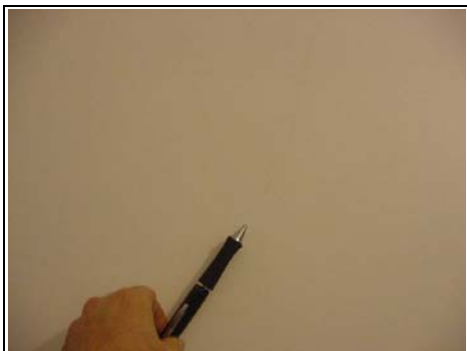
An example of the hairline cracking
