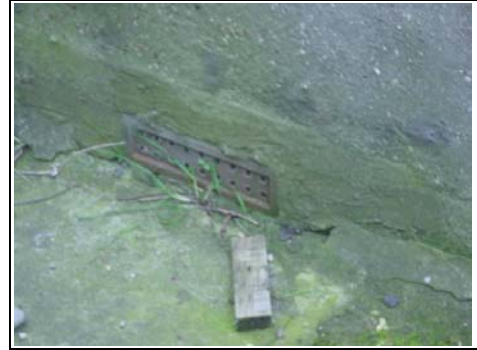
Air vent acting as a gully
