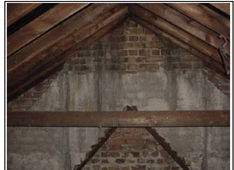
Pattern staining indicating that dampness is coming through the cement flashings
