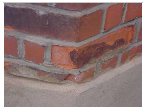
Spalling red brick
