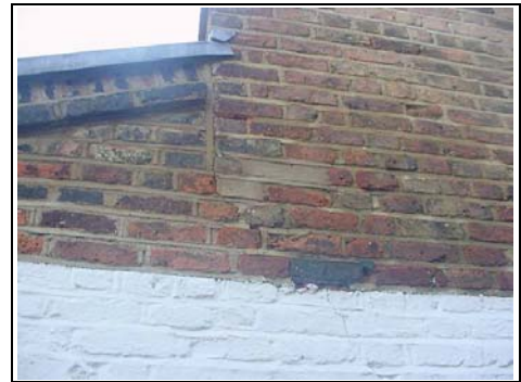
Your neighbour's wall with a crack where it has been extended
