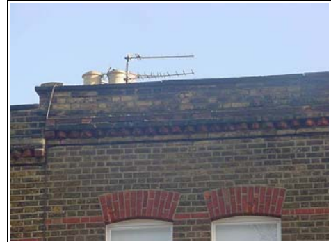
Defective Parapet Wall to the front of the property which is allowing dampness in to the front wall.
