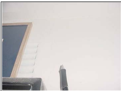
An example of the hairline cracking to the rear wall of the bathroom
