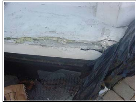
De-lamination of Bay Window Sill
