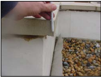
Where mastic drip has been added
