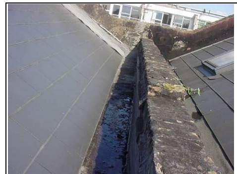
The parapet wall that is allowing water in. This explains the plant growing out of it. This needs to be made watertight
