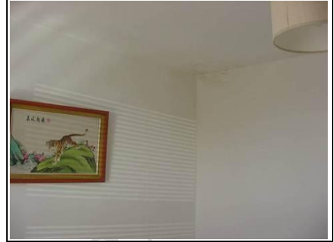
Dampness in the corner of the rear bedroom
