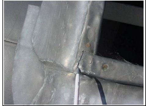
Damage to the lead
