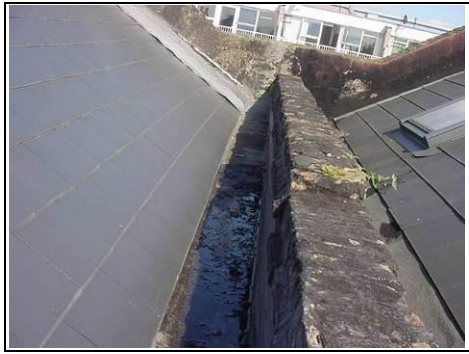
Valley gutter to the left hand side (all directions given as you face the property). Ponding is visible on it.
