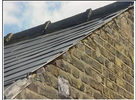
Close up of flashing put on incorrectly
