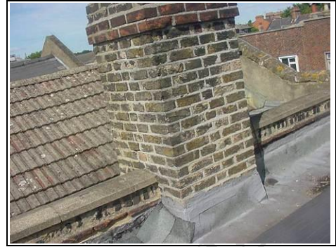
The chimney has felt flashing around it
