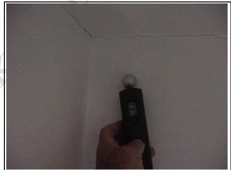
Reading of 33 on the Gann meter. This is acceptable but the hairline cracking does suggest something has occurred
