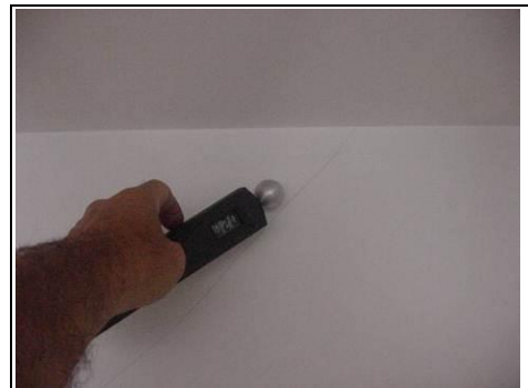
Hairline crack with reading of 28
