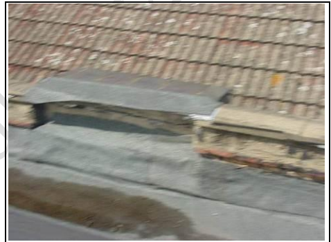
Chimney has been removed with a felt capping in place rather than a paving slab or concrete.
