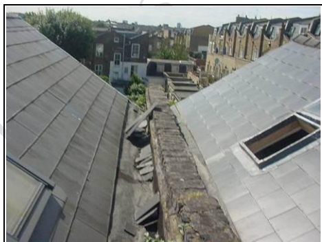
Many slates have been damaged
