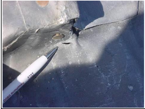
Split lead to the access area
