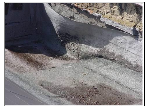
Felt flashing that is coming away. Lead should have been used.
