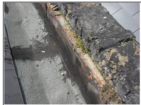
Bitumen repair. Also note the parapet wall is letting in water which is why the plants are growing from it
