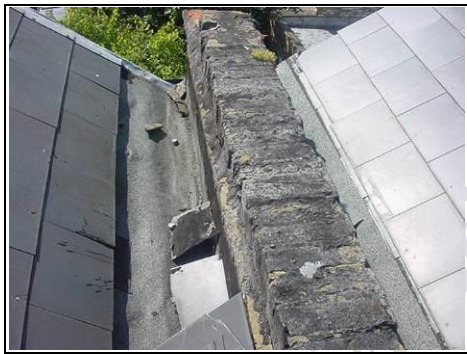
This could affect you as it is in poor condition with the felt becoming un-bonded
