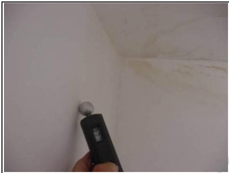
Damp meter reading of 77
