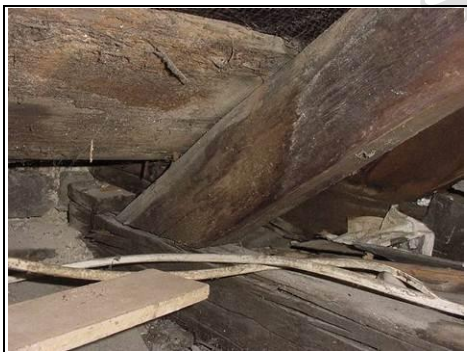
Staining on the timber that is typical from what you see from a leaking valley gutter
