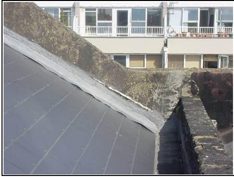
Flashing to the front that's not bedded properly
