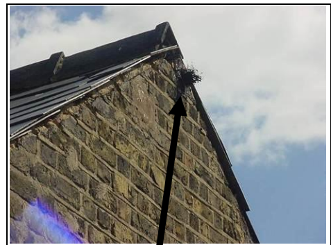
Vegetation growing from the top of the gable
