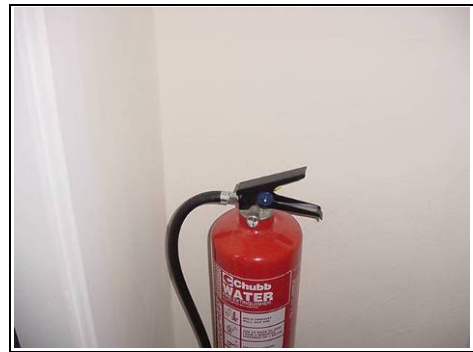
Fire extinguisher not identified.
