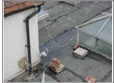
Water sitting on the roof
