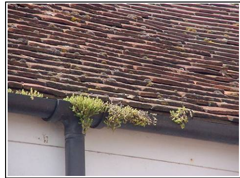
We would expect the fascias to be deteriorating where the gutters are blocked.
