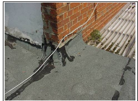
Poor flashing detail and blisters to the felt
