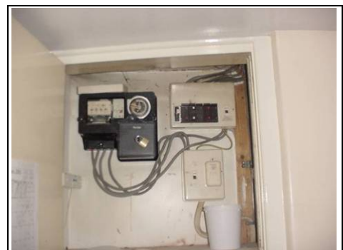
1960s fuse board on the top floor.
