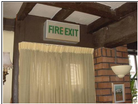
Old style fire exit sign needs changing.
