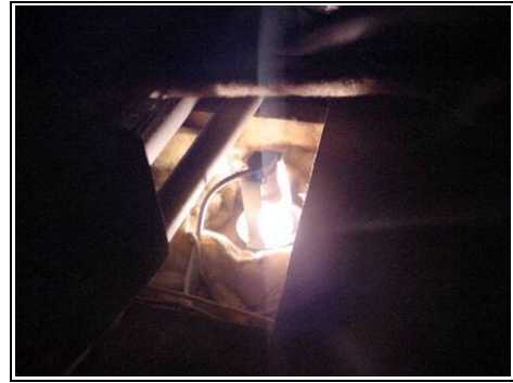
Back of ceiling light
