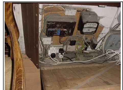
1960s ground floor fuse board
