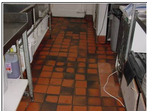
Tiles need a good clean
