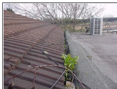
Awkward roof/guttering detail to the top
