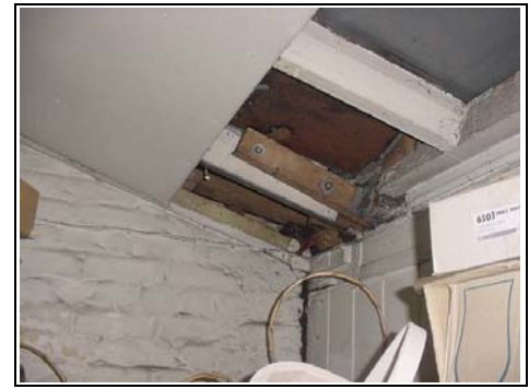
Deteriorating roof timbers / common rafters. We can also see other areas of timber deterioration.
