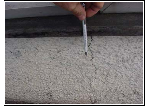
Vertical crack under window
