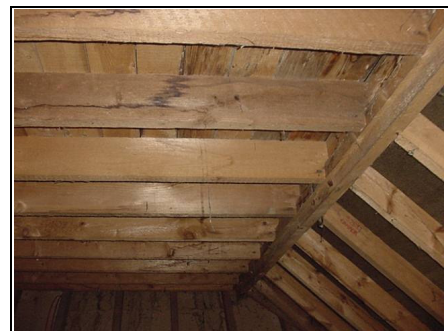
Dampness getting into flat roof near ballroom
