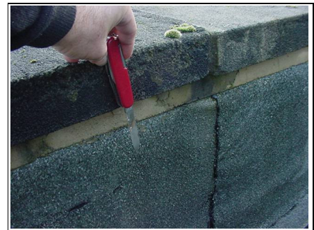
Parapet wall without suitable drip
