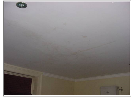
Visible leak to ceiling
