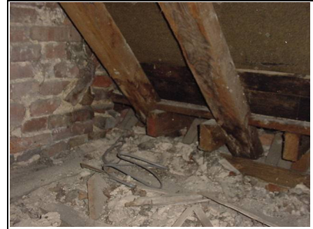
The darker areas are the deteriorating timber
