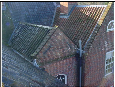
Awkward valley gutters
