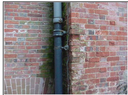
Dampness on the walls
