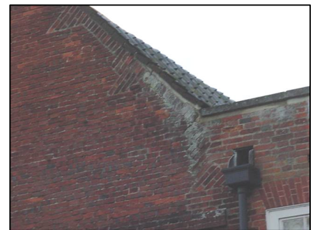
Damage to brick parapet wall
