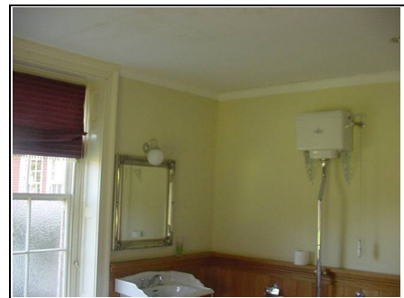
Leaks in corner of room come from the valley gutter above
