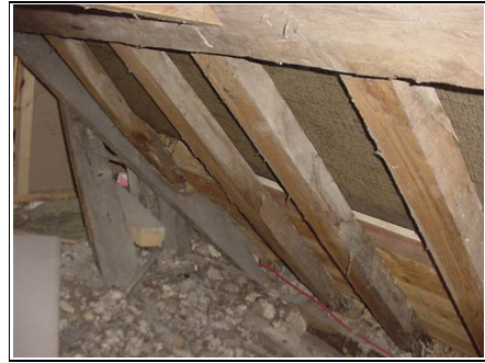
Staining to the timbers indicating dampness getting in.
