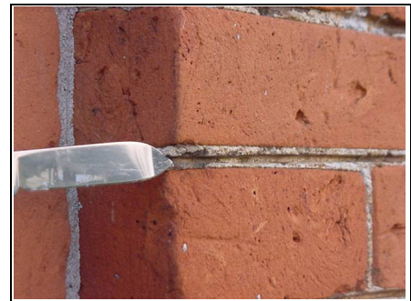
Re-pointing required to pinch pointing
