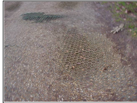
The parking area needs some work
