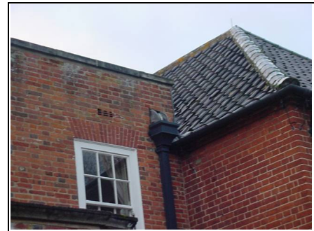
Air vent located above window
