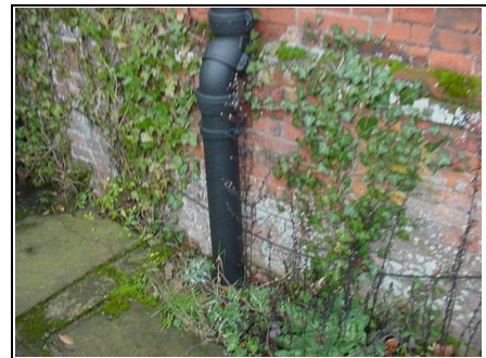
Relatively new soil and vent pipe
