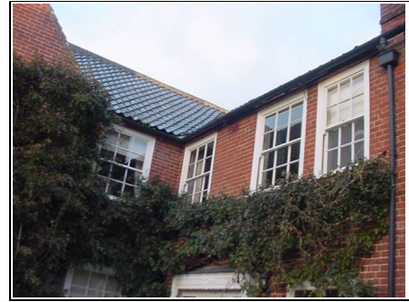
Vegetation needs cutting back
