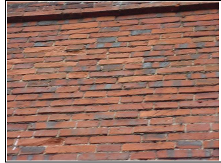
Deterioration to soft red bricks
