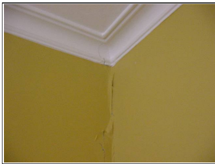
Differential movement in Traffords room between the bedroom and adjoining corridor
