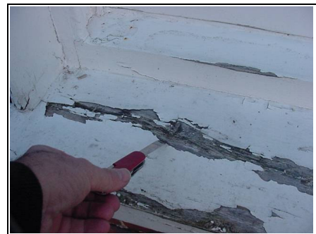
Close up where the rot is not as bad as we expected when tested with a knife sliding sash window
