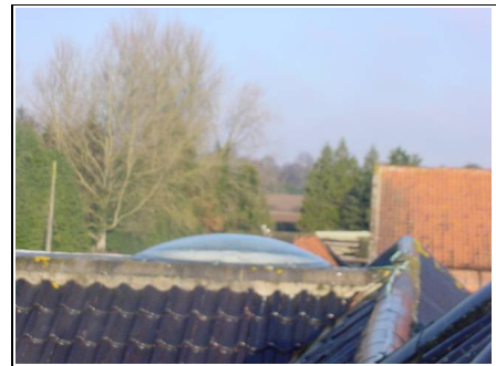
Manufactured dome roof light over ballroom staircase
