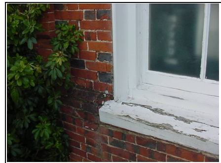
General view of deteriorating sliding sash window
