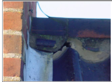
Damage to the side of the chimney which needs repair
