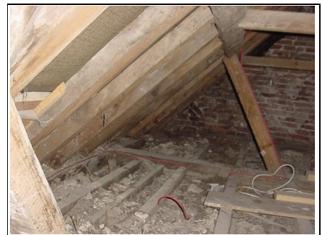
Dampness in the roof space beneath the awkward valley gutter
