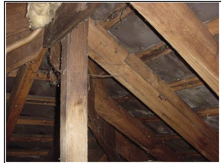
No protective underlayer
