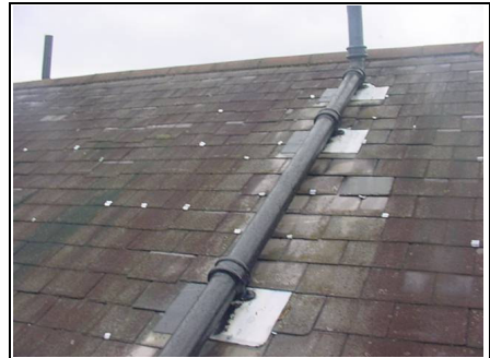
Soil and vent pipe
