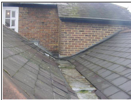
Water sitting on roof
