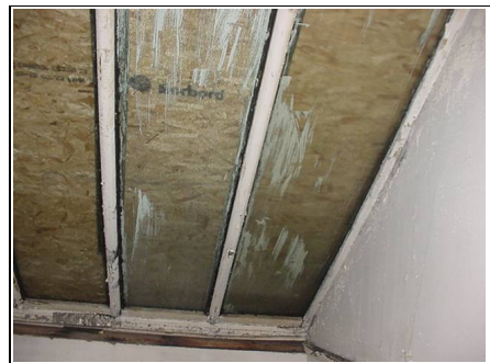
The underside where you can see the timber that has been put over the roof window
