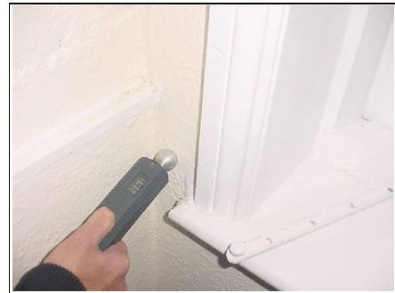
Checking for lateral dampness
