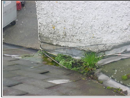
Left hand side valley gutter full of vegetation
