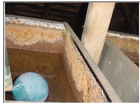
Rusting water tank
