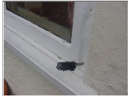
Deterioration to timber windows
