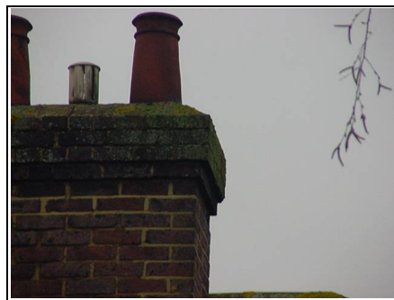
Close up of rear chimney in need of repointing. Note the moss to the flashing (top of chimney)
