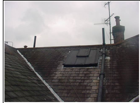
Tarred over skylight
