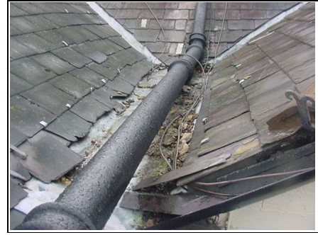
Debris in the valley on right hand side
