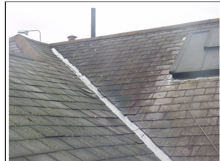
Close up of high level main roof. Note lead tingles and our comments on these.
