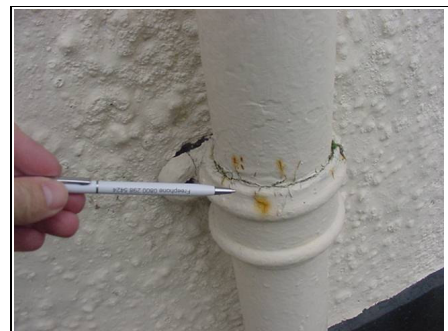
Rust coming through
