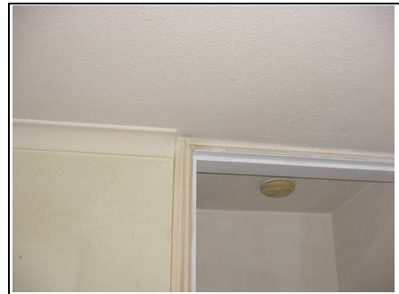
Nicotine staining to left of photo
