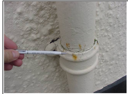
Rust to cast iron gutters and downpipes
