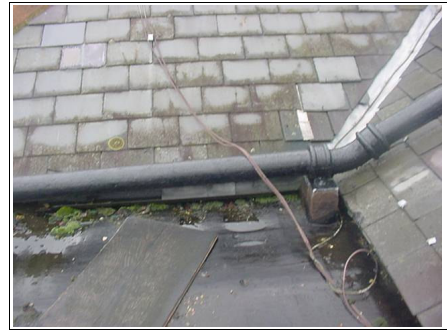
Moss sitting on roof on left hand side
