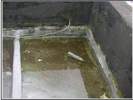
Flooded front left flat roof
