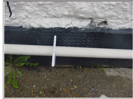
Air vent to left hand side
