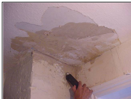
Damage that has been caused within the building from the leaking large rear chimney
