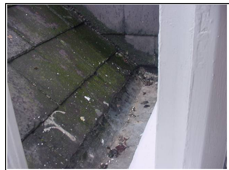
Valley gutter to right hand side with water sitting against the building allowing damp in
