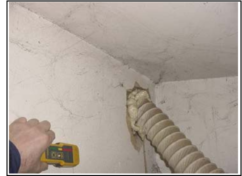
Testing for lateral damp
