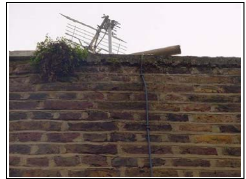
Plants growing out of parapet wall on next door's property
