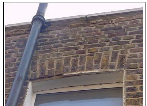
Close up of parapet wall showing repointing and some spalling to the brickwork at the top
