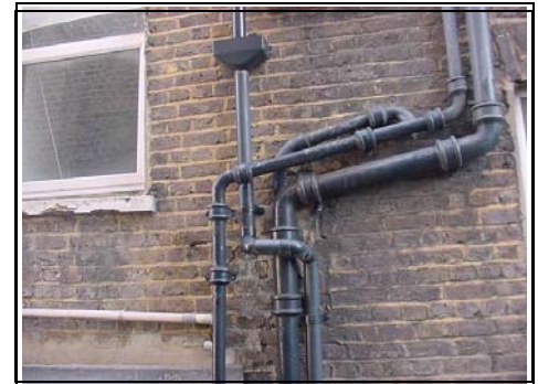
We can see a mass of pipes to the rear of the property
