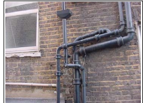
We can see a mass of pipes to the rear of the property
