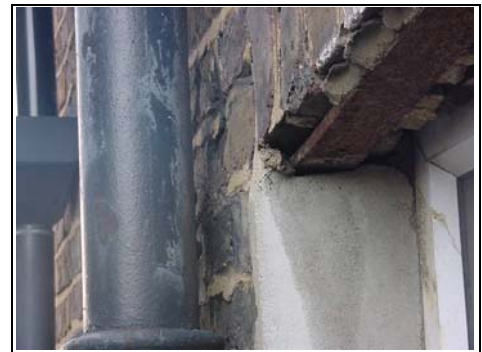
Repairs to one of the windows due to movement
