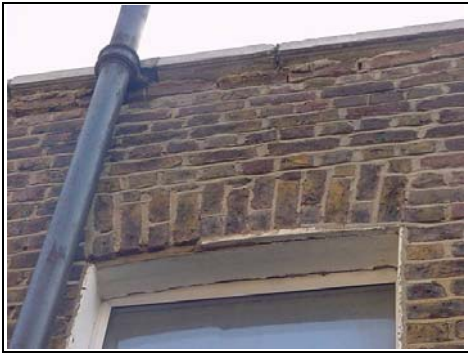
Repointing and deterioration above the window onto the parapet walls brickwork and associated pointing
