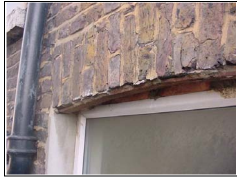
This photo shows lintel repairs in the form of a metal plate lintel
