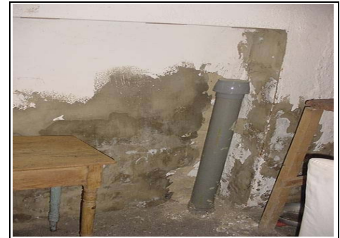
The soil and vent pipe is on the right hand side
