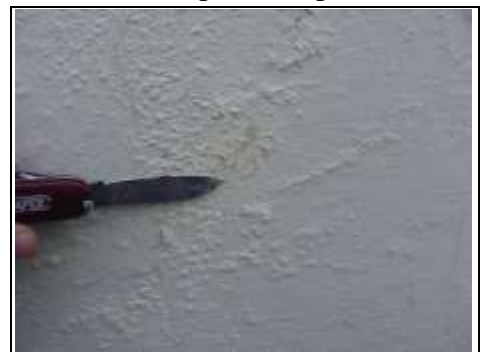
Deteriorating render through dampness
