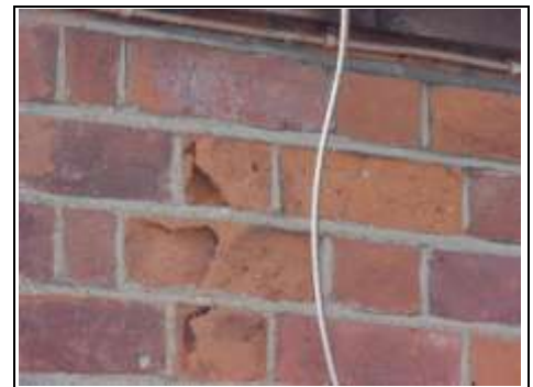
Wrongly repointed in cement mortar
