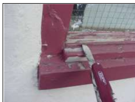
Rot to windows
