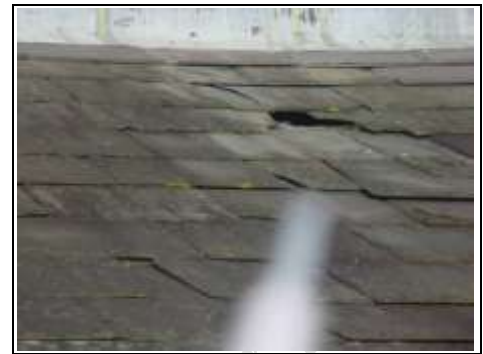
Slates completely displaced.
