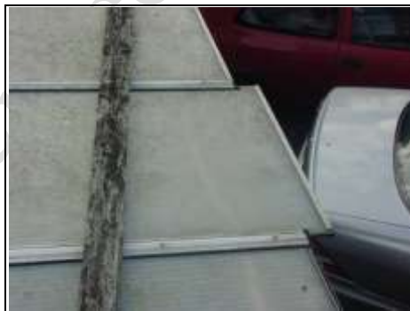
Some polycarbonate panels are out of place
