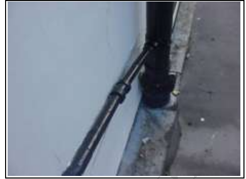
Plastic soil and vent pipe
