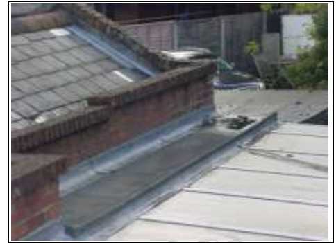
Small flat roof to the link section between original building and conservatory
