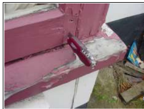
Rot to windows
