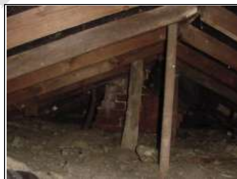
Dampness visible to central chimney
