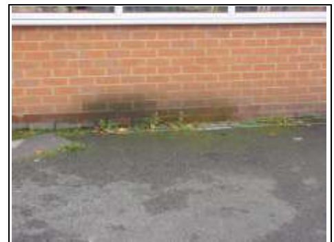
Water discharging against building
