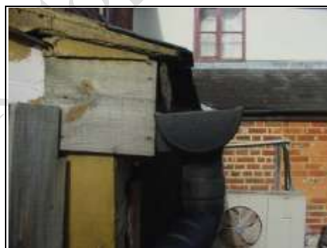
Fascias and soffits not painted at all
