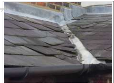
Slates in mess to high level roof
