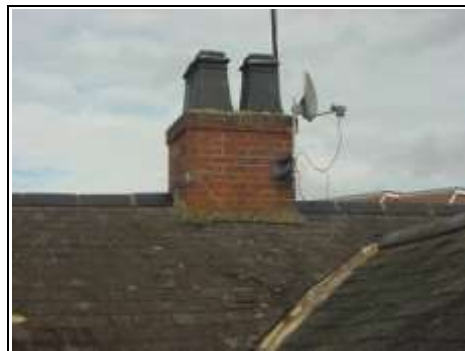
Cement flashing to middle chimney allowing dampness in
