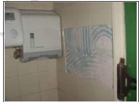
Blown tiles to walls
