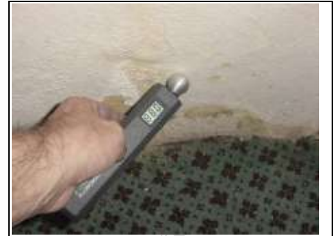
Dampness in bar
