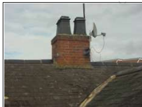
Cement flashings on middle chimney, replace with lead
