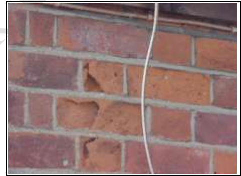
Wrongly repointed in cement mortar
