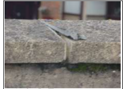
Part of parapet wall coping stones have been masticed in place due to leaks
