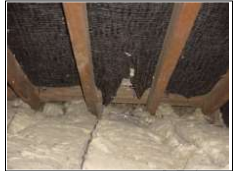
Damage to sarking felt
