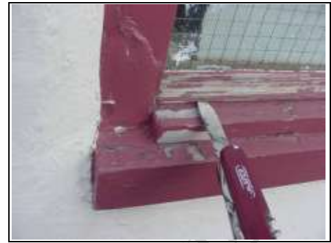
Bare timber visible and some rot to windows
