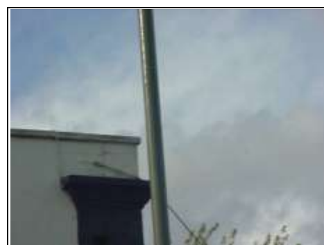
Hopper head to left hand side of property leaking and paint flaking
