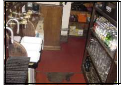
Worn altro style floor in bar
