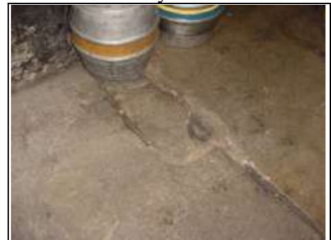
Cracked and uneven floor to cellar
