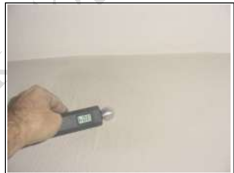
Testing for lateral dampness within rear right hand bedroom
