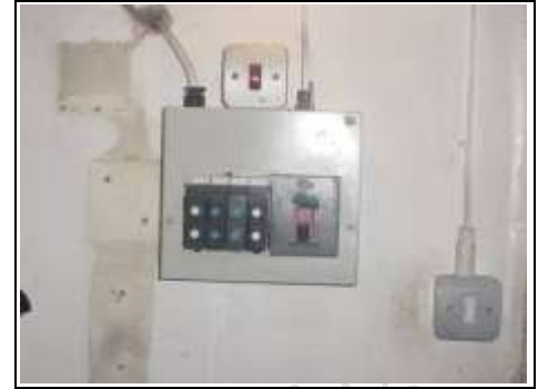
Old fuse board
