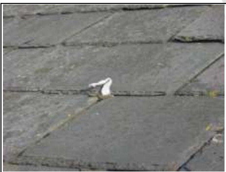
Tingles on slates
