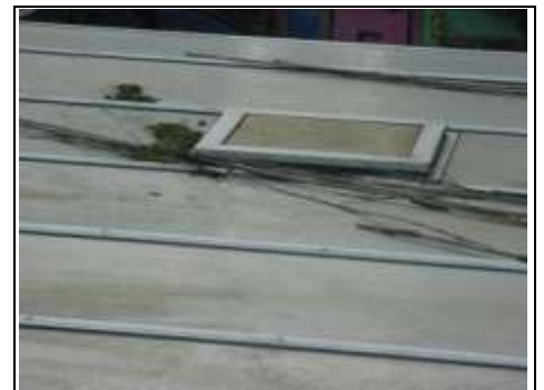
Vent in polycarbonate roof which we were pleased to see as it will get heat gain in the summer and heat loss in the winter
