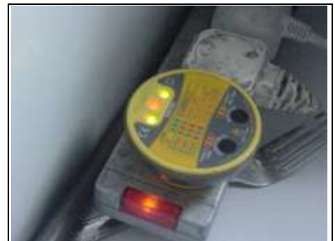
Earth test failed
