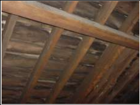
Dampness coming through the roof
