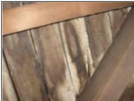
Signs of dampness to boarding
