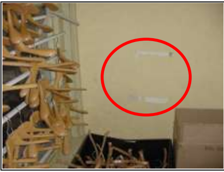
Heavily marked wall in store room
