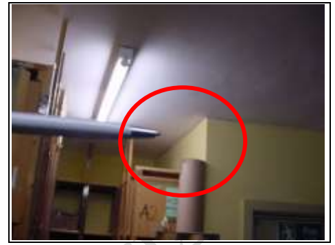
Cracks between studwork partitions and ceilings
