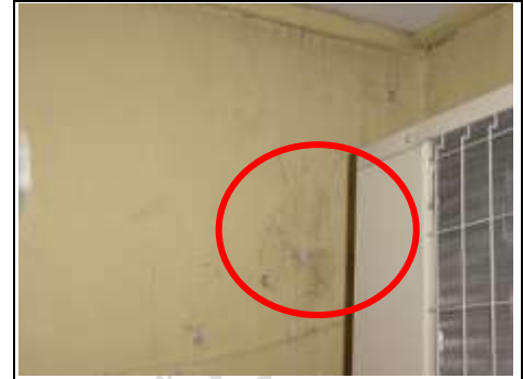
Dampness in plant room
