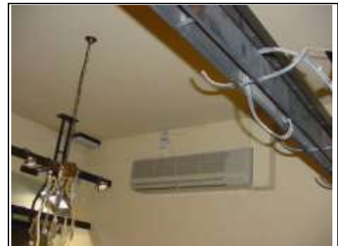
High level heaters
