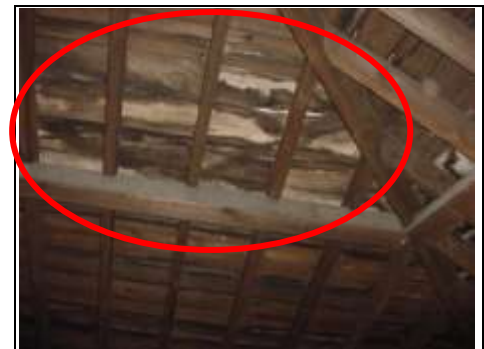
Dampness coming through close boarding
