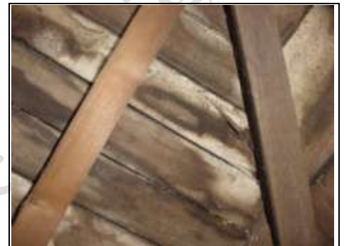
Dampness to boarding
