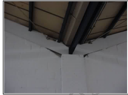
Rusting, indicating dampness getting in
