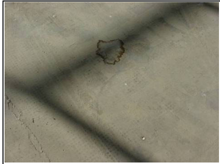
Staining on concrete floor
