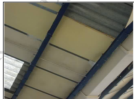
Different colour under cladding where it has been changed
