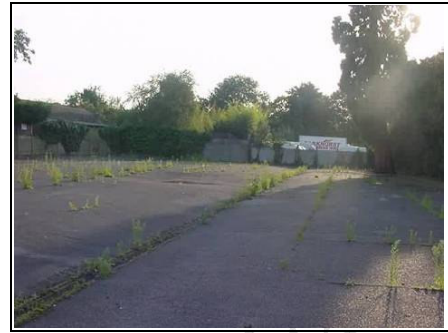
Car park deteriorating
