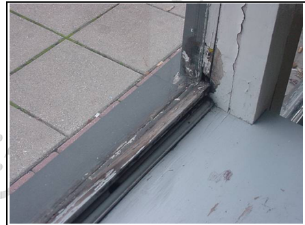
Flaking paint to window cill
