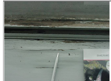
Pen indicates deterioration to timber window to front
