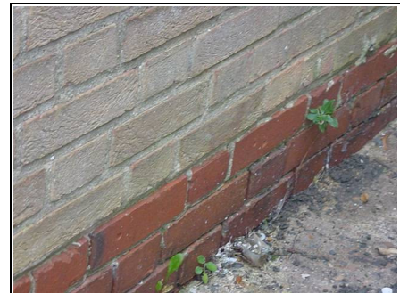
Weathering to brickwork
