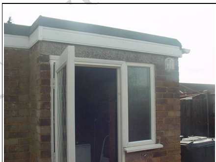
Example of a concrete lintel – can you notice where the cold bridging would be in this photo?
