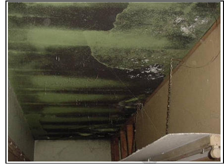
Salt coming through ceiling
