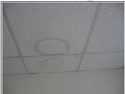
Leak staining visible in ceiling tiles
