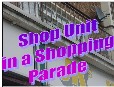
Dampness coming through the front balcony above shop
