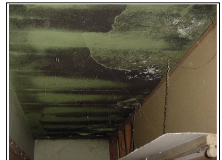
Salt coming through ceiling
