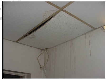
Ceiling coming down due to dampness / a leak
