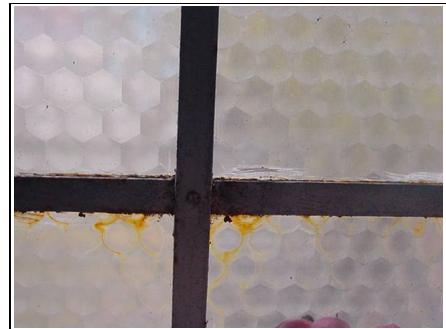
Rusting rear metal windows
