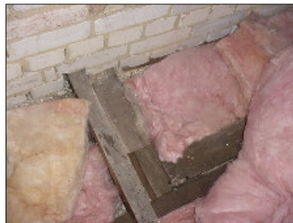
Here we tried to clear some of the insulation to have a look at the timbers, but there was a lot of it and it was not practicable to clear.
