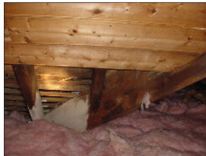
You can see the darker bits of timber, where there is some dampness getting in.
