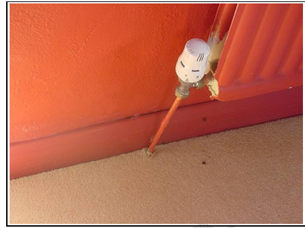
Micro bore pipes
