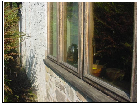
Window in need of repair and redecoration
