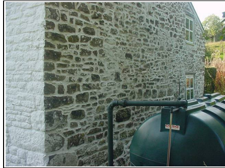
Defective wall coating
