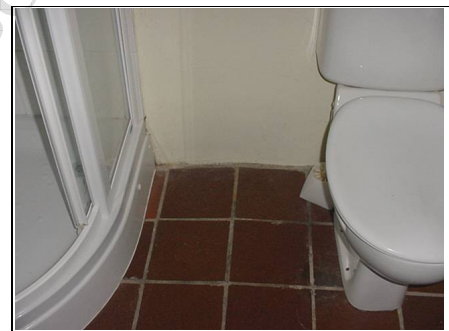
Lifting off the floor which we believe relates to dampness
