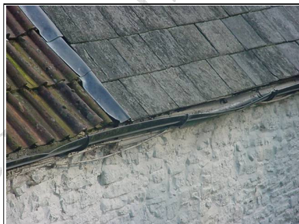
Defective guttering and downpipe
