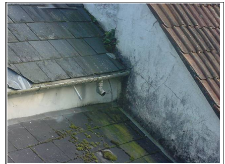
Rear left hand side slate roof – in worst of conditions which looks to have some man made slates
