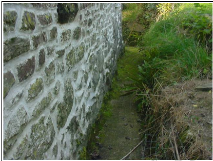
Gulley behind shower room area
