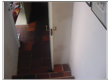
Dampness found around the steps down into the kitchen area
