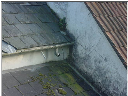
Dampness coming in via step in roof
