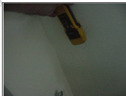
Rising damp in rear shower room
