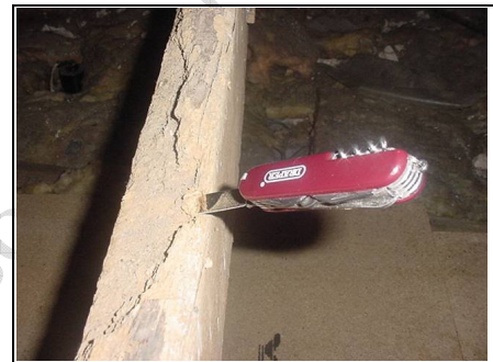
Woodworm in roof over right hand bedroom
