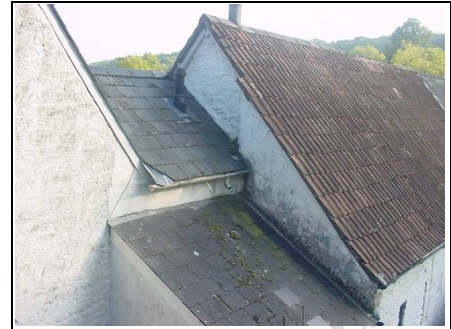
Dampness to upstand
