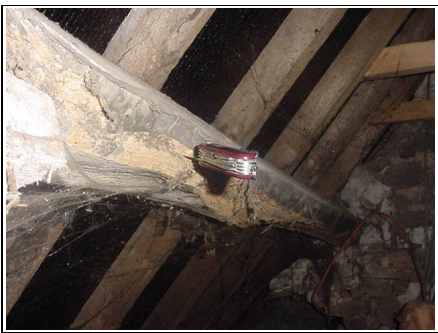
Third roof where there is the worst woodworm
