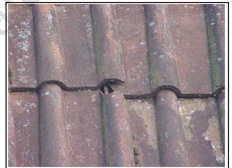
Damage in tile of roof
