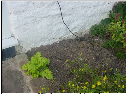
High ground level
