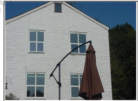
Crack not visible to outside of property due to paintwork
