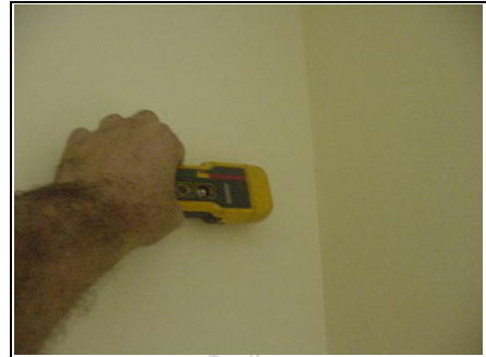
Dampness found to chimney breast in right hand side of property
