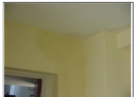
Damp staining to right hand side of property which we believe is coming from a leaking roof or leaking soil pipes
