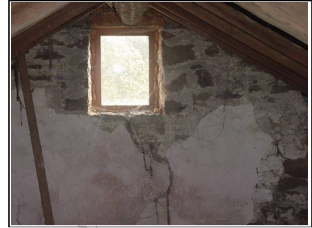
Crack to front right hand gable
