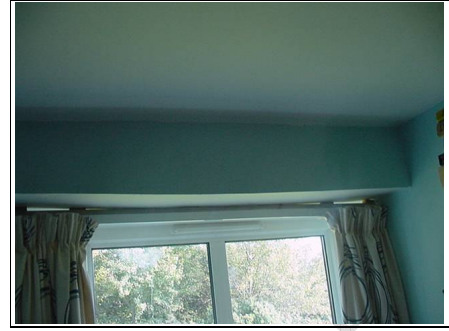
Dip in lintel
