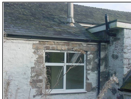
Soil and vent pipe
