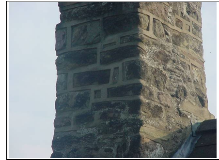
Close up of cement repair to main central chimney
