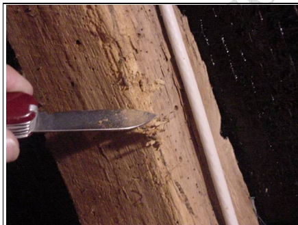
Woodworm in roof over kitchen – frass on top of knife
