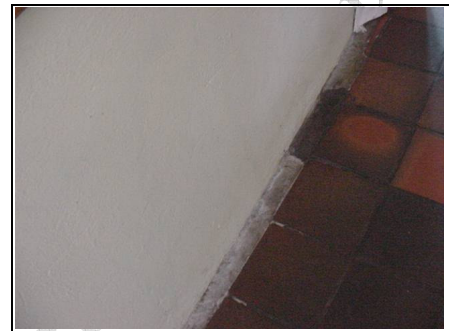
Poorly finished kitchen tiles
