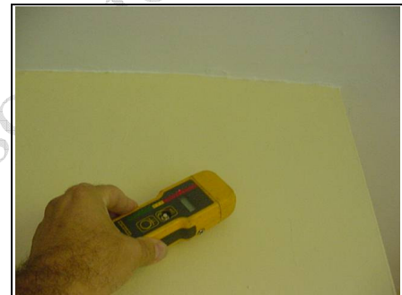
High level damp internally in far end of property
