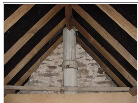
Water staining on flue indicating dampness is getting in
