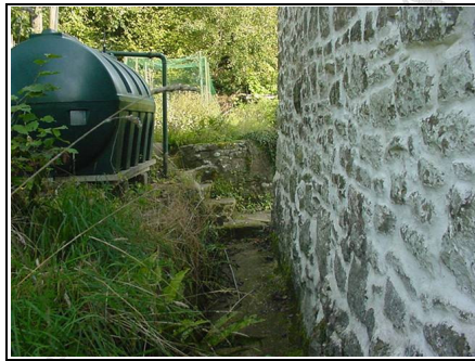
Dampness coming in through the rear wall at ground level where you can see the moss and due to the lack of a protective coating to the walls
