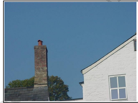
Badly repaired chimney
