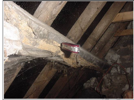
Utility/services room roof which is in a poor structural condition due to woodworm
