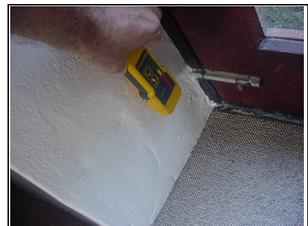
Dampness found by door in lounge with feature chimney
