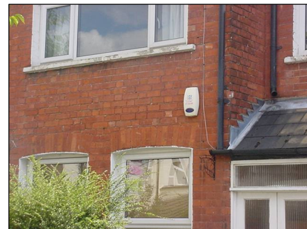
Brickwork needs repointing
