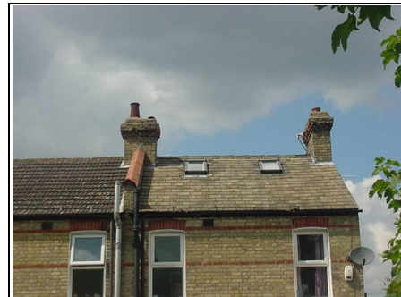
Fascia board hidden by guttering
