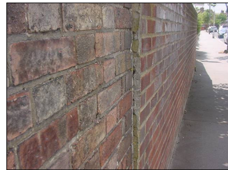
Movement in the neighbours' wall
