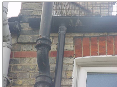
Soil and vent pipes
