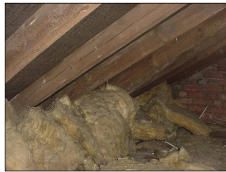
A split in the timber and also some dampness of the timber.
