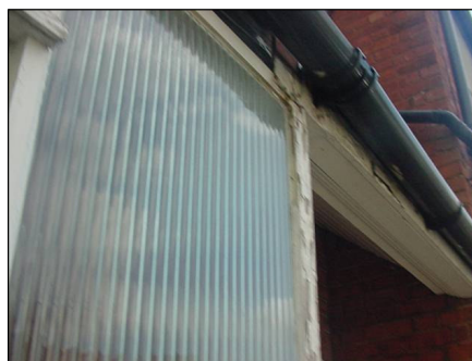
Timber surround in need of redecoration
