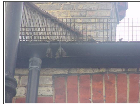
Minor leaks can be seen on the gutter
