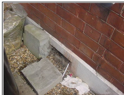
Airbricks to front being blocked
