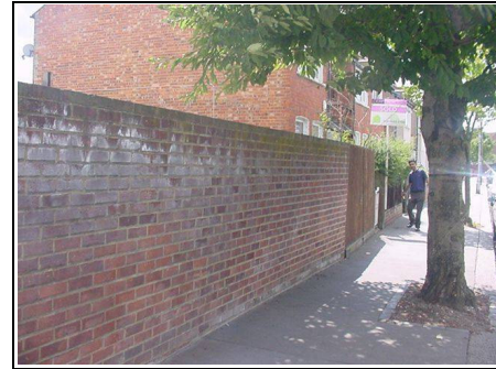
Neighbours wall moving, LHS of your house
