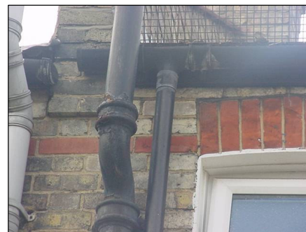
Leaking gutter and downpipe and rusting cast iron soil and vent pipe.
