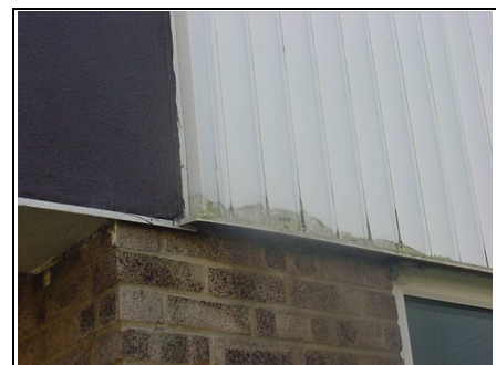
Some deterioration to base of cladding
