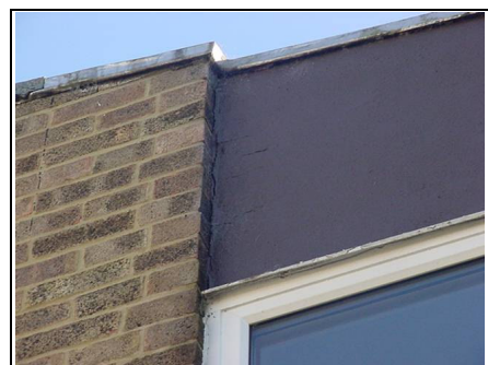
Mastic going between render and brickwork
