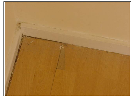
Damage to timber floor
