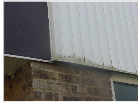
Deterioration to base of cladding board
