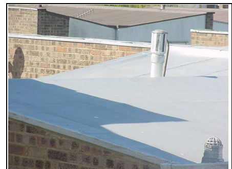
Soil and vent pipe in front right hand corner and asbestos flue pipe in rear
