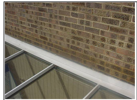
Lack of flashing to conservatory roof
