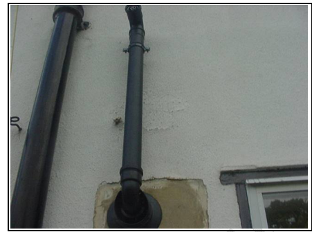
Flue from boiler
