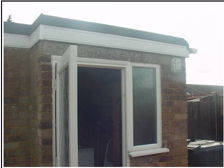
A rear door to a 1970's building. Can you tell where the cold bridging would be in this photo?
