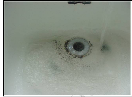
Deterioration to kitchen sink – needs replacing
