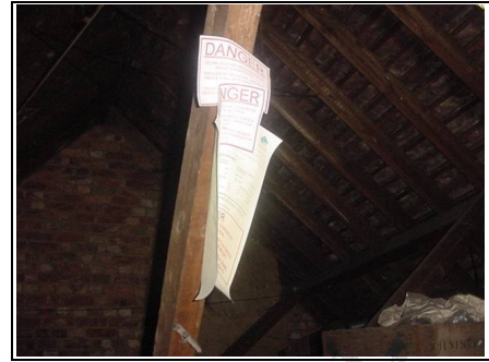
Danger notice – mass of insulation
