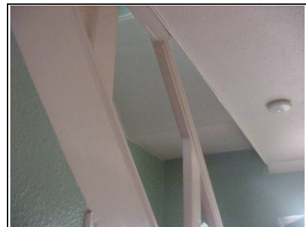
Handrail openings on stairs are wider than is now acceptable.
