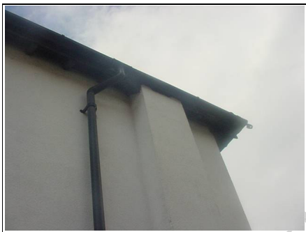
Plastic gutters and downpipes
