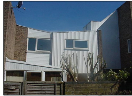
1970's property with cold bridging to the roof beams and the lintels
