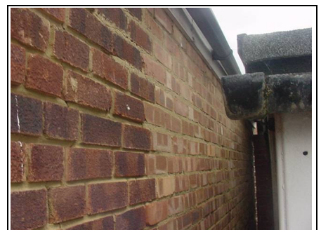
Next door's wall on right hand side would benefit from being tidied up
