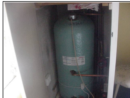
Hot water cylinder
