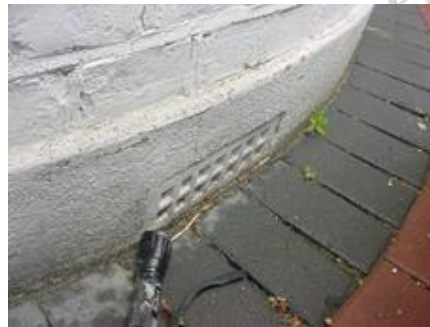
The brick pavers too high
