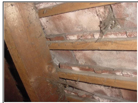
Close up of back of tiles, lighter areas are where dampness is getting through
