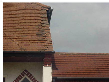
Distortion of tiles
