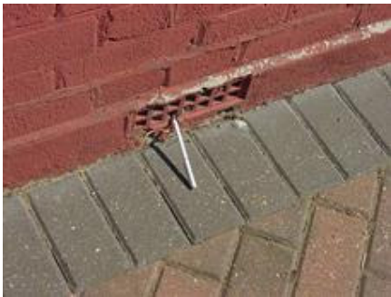
Airbrick allowing water into the building
