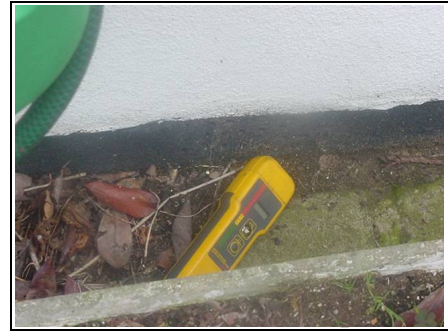
Airbrick to rear not adequate
