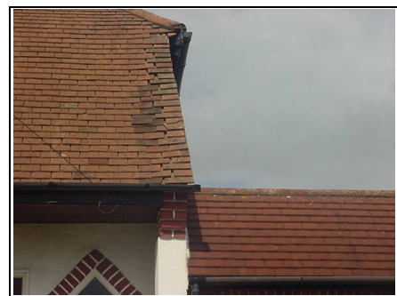
Distortion of tiles
