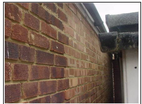
Cast iron gutter to rear of garage
