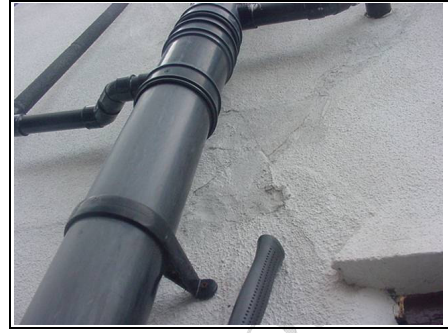
Soil and vent pipe
