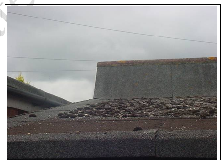
Moss on flat roof
