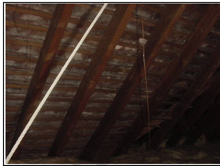
Back of tiles exposed
