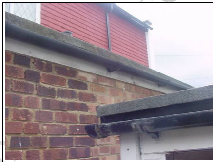
Gutter to the garage looks like it is leaking and hasn't got a fall on it towards the downpipe
