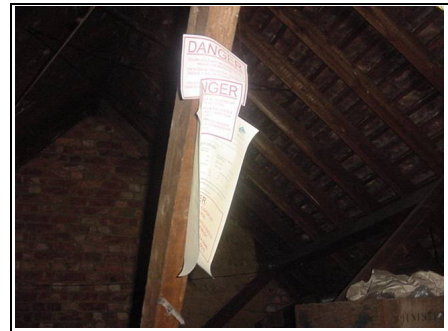
Danger notice – mass of insulation
