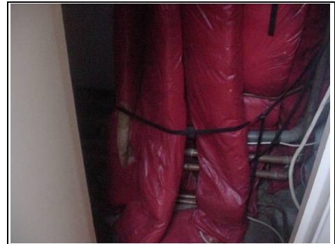
Hot water cylinder
