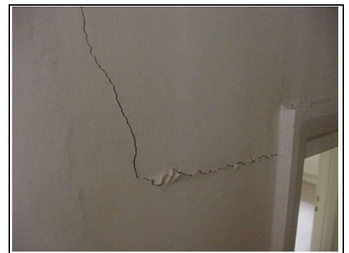
Cracking near the stairs to the top floor
