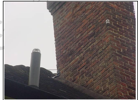
Plastic soil and vent pipe
