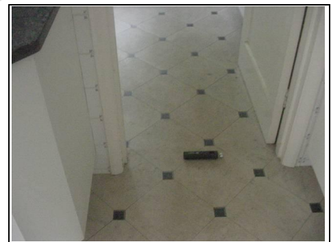
Start of suspended floor to the rear with concrete floor at the front
