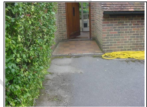
This is where the water runs to and sits.
