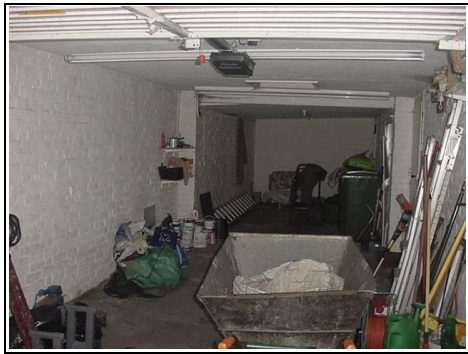
Dampness in the garage
