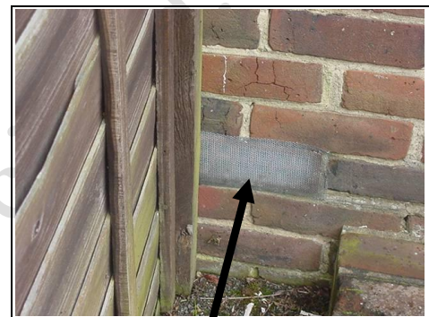
Air brick with grill over it
