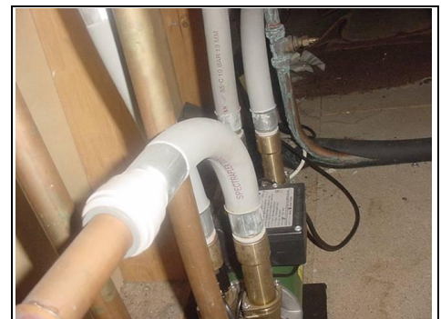
Plastic and copper pipes
