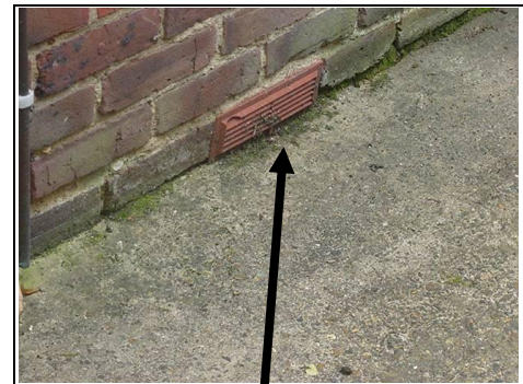
Plastic air brick rear left hand side
