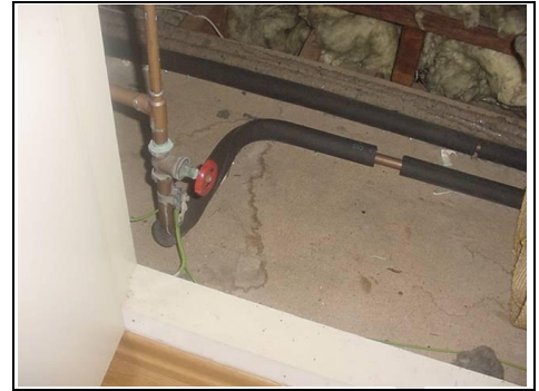
Leaks in the plumbing
