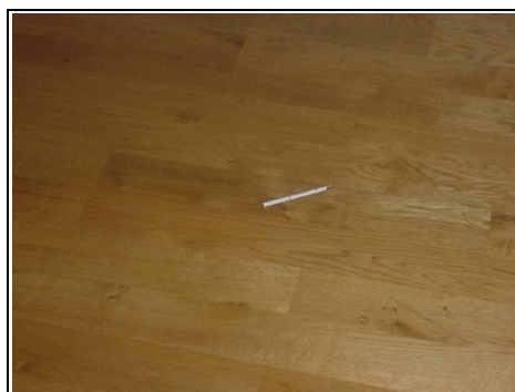
Spongy area of the floor marked by the pen
