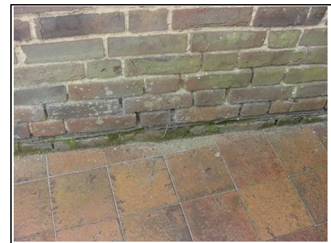
DPC is too low in some areas
