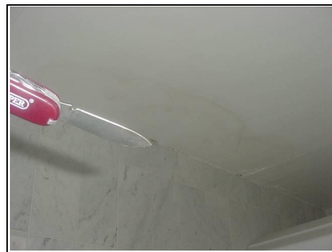
Leak in the top floor bathroom
