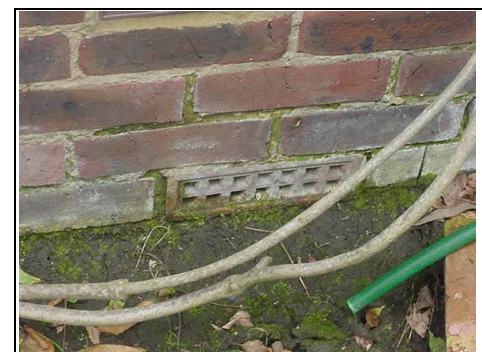
Air brick needs clearing
