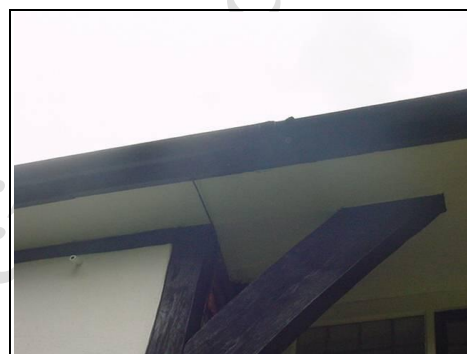
Leaking gutter (front)
