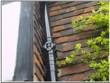
Plastic soil and vent pipe
