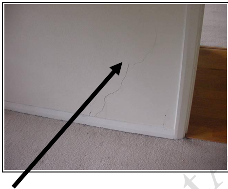
Cracking in first floor front left bedroom
