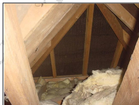
Mass of insulation may cause condensation
