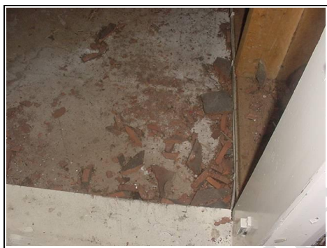
Broken tiles that have been replaced before
