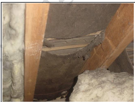
Deteriorating builders felt
