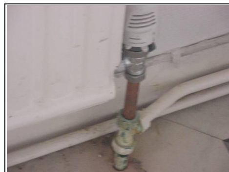
Copper pipe visible and rusting to the joint
