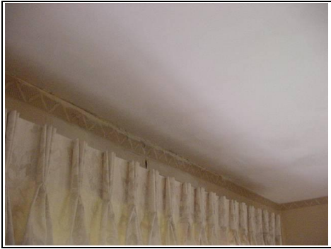
Old leak visible on ceiling. This has now been resolved
