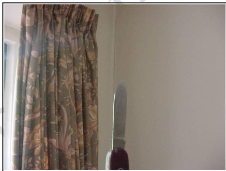
Cracking in the corner, front left hand bedroom
