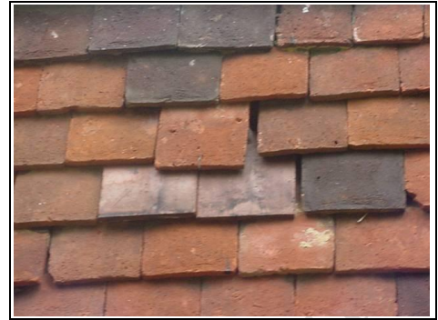
Slipped tiles and mismatched tiles
