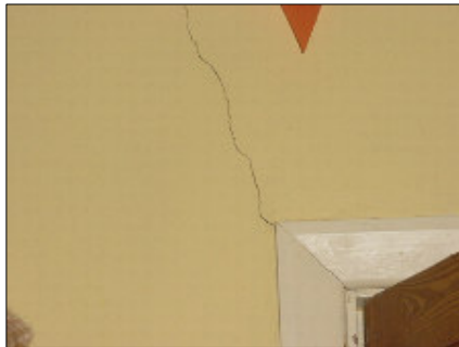
There is a hairline crack to the wall in the front right hand small bedroom.
