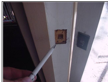
Missing door closer
