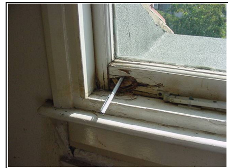
Rotten window to the dormer at the front of the property
