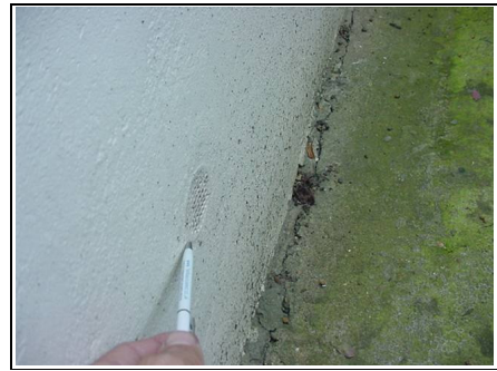
This is an air venting system that does not tend to work. We would recommend that a bell mouth detail is added to the base of the render
