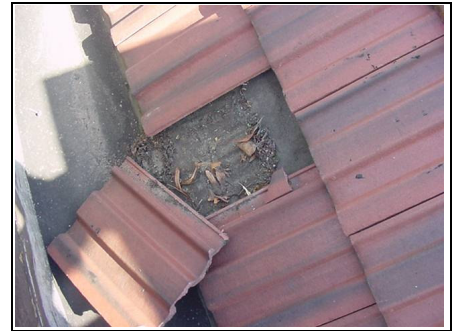
Displaced roof tile (which we did put back in place)
