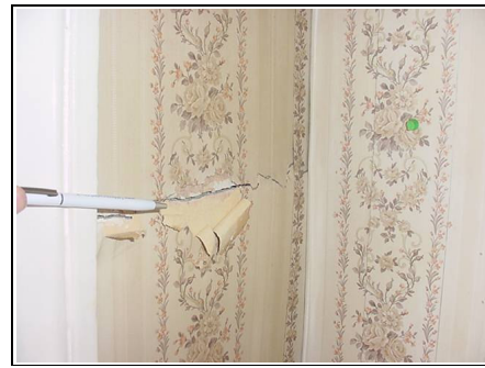
Cracking on wall
