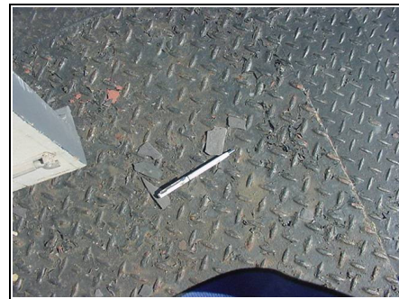
Rusting fire escape
