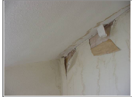
Dampness to the rear of the property on the top floor
