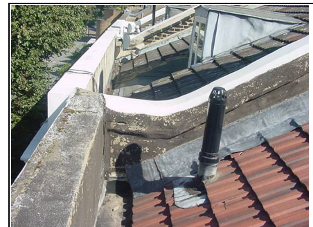
Soil and vent pipe
