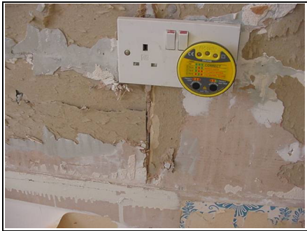
Earth test in kitchen, which failed
