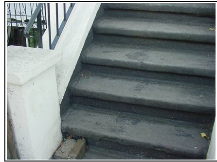
Asphalt covered entrance steps
