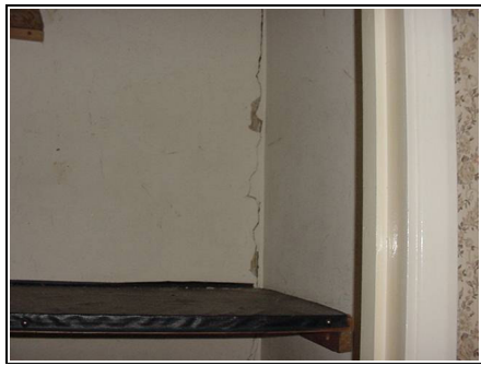
Cracking caused by movement
