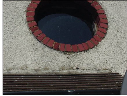
Cracking to the rear render really concerns us.
