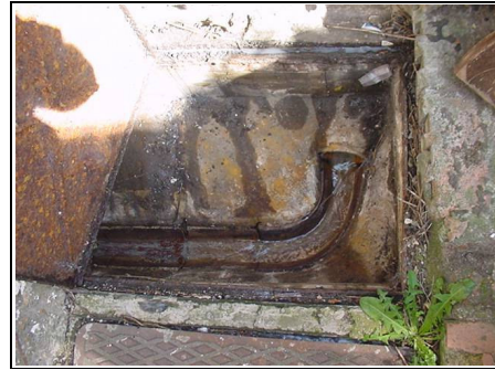
Rear left hand side drain with signs that it has been overflowing
