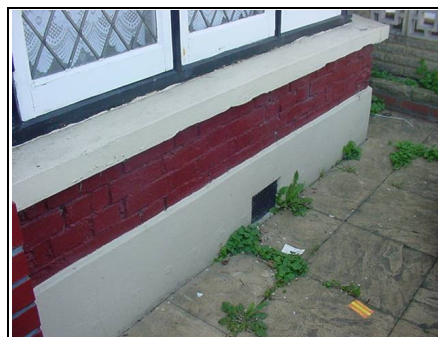
Render obscuring view of damp proof course
