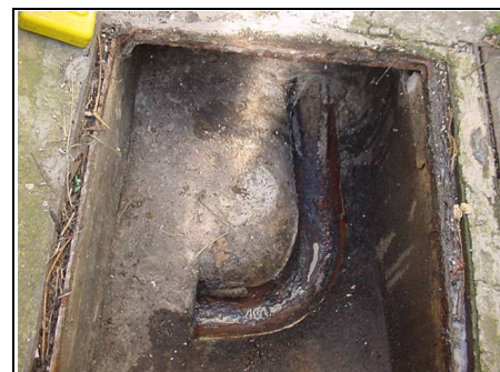
Rear right hand drain
