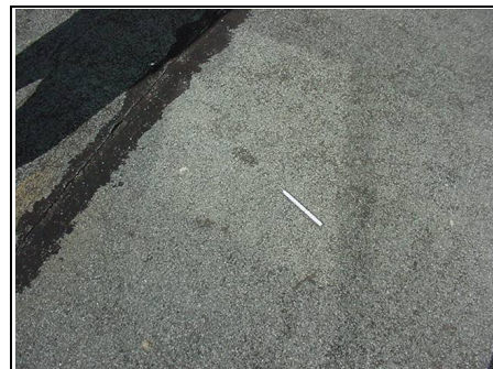
Blistering to roof
