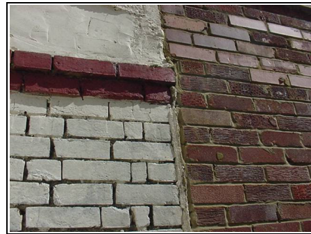
Brickwork needing re-pointing in appropriate mortar
