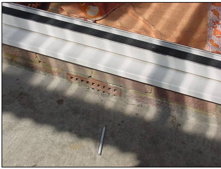
Rear airbrick partially covered
