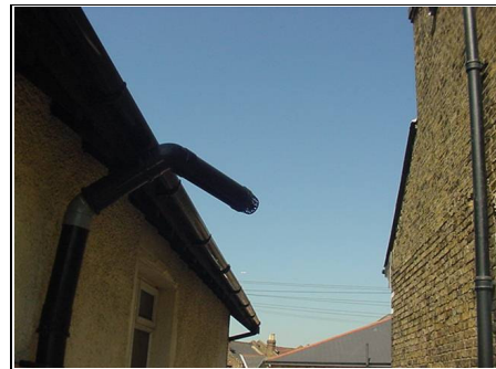
Soil and vent pipe should be pointing upwards
