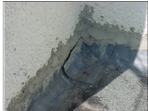
Poor quality lead flashings
