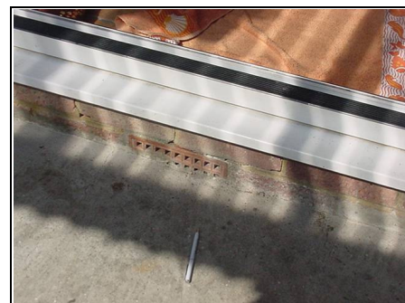
Airbrick at rear partially covered
