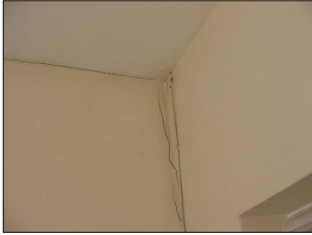
Close up of the cracking to the wall between extension and original building
