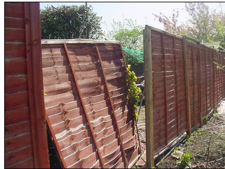
Fence needing to be secured/repared
