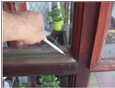
Wet rot in timber
