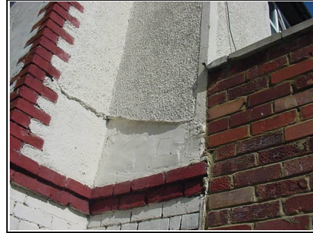
Cracking to the render
