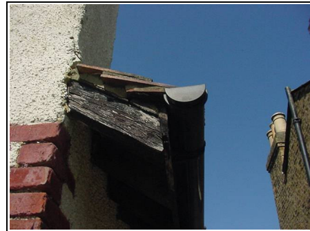
Fascia boards in need of redecoration although most hidden behind guttering
