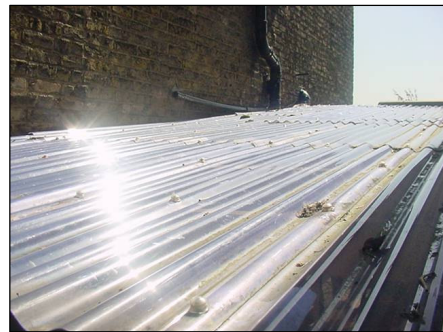
Two sides of roof discharge onto neighbour's property
