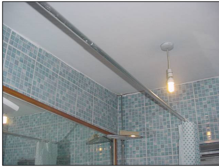
Movement between wall and ceiling in the first floor bathroom
