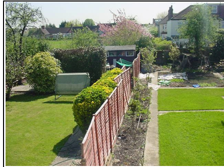
Rear garden fence to left hand side in need of securing
