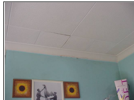
Polystyrene ceiling tiles
