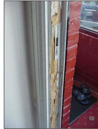
Damaged front door
