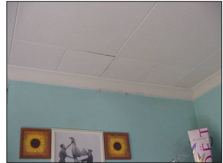
Dampness coming into the rear right hand chimney
