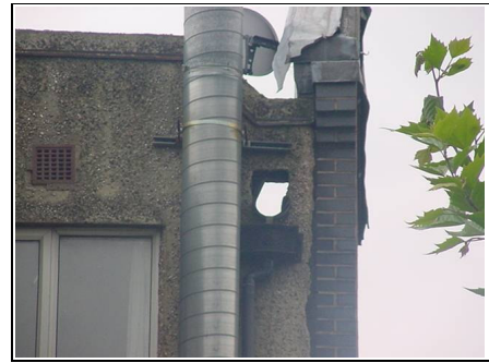
Cast iron hopper head into plastic downpipes
