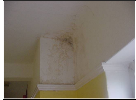
Dampness coming through
