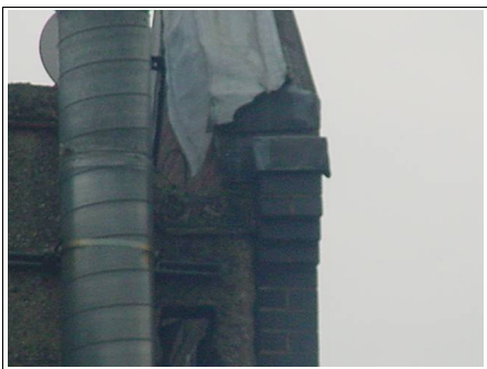
Flashing hanging off parapet wall
