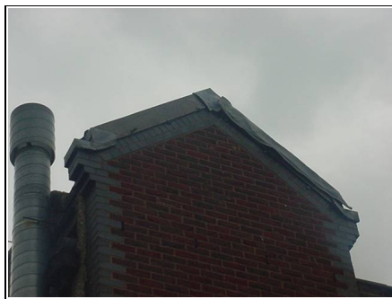
Missing lead coping On left hand side
