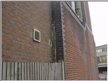
Staining to brickwork indicating dampness
