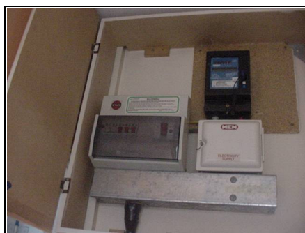
Fuseboard on first floor
