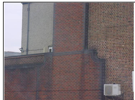
Pattern staining/ dampness getting into walls
