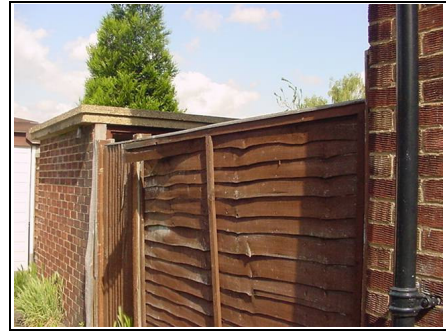
Fence falling down
