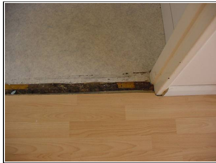
Laminated flooring – fitted badly
