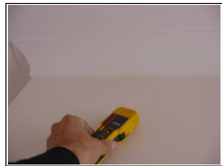
Checking for lateral damp
