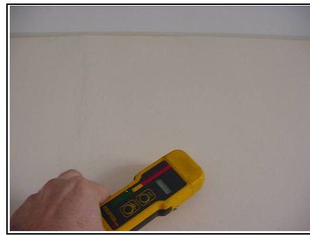
Checking for Lateral Damp
