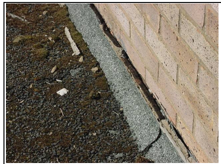
Flashing coming away
