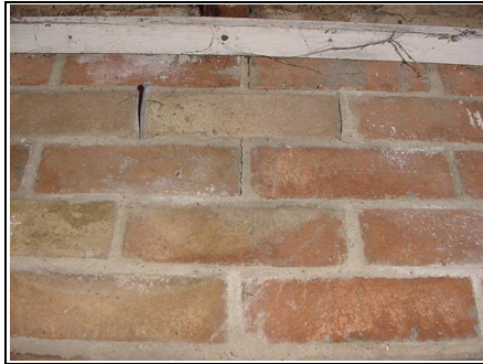
Single skin brick wall opening up - note the vertical cracks.
