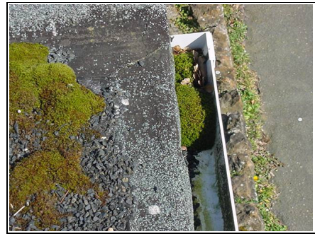
Low level guttering blocked with moss
