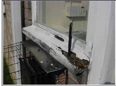
Rotten window to the rear next to the garage.
