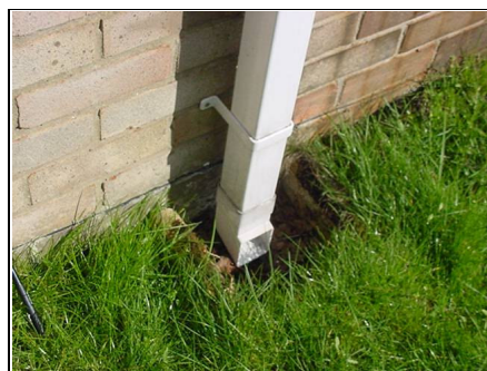
The gully is blocked with leaves and needs clearing.
