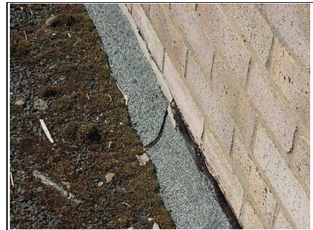
Flashing coming away.
