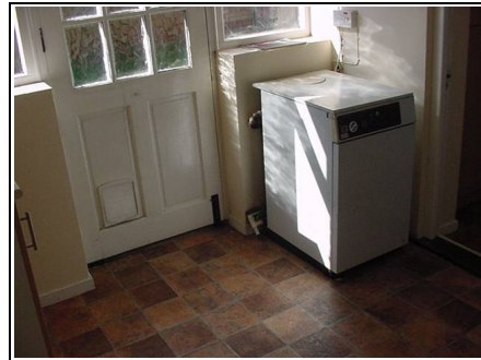
Utility Room and boiler
