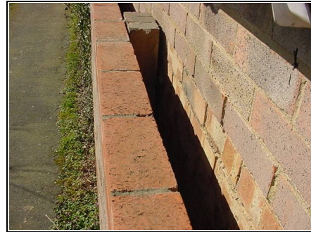
The right hand wall in this photo is the one with the cracking
