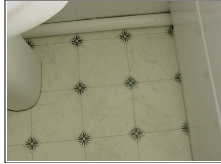
Puddle of water on the floor
