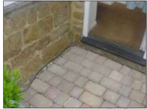
Outside ground level to close to inside ground level
