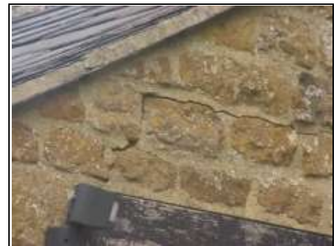
Cracking in outbuilding
