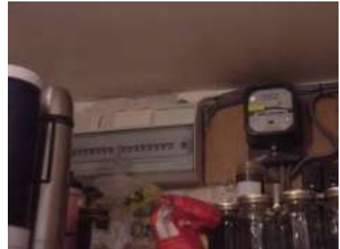
Electric fuse board
