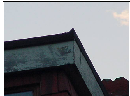
A close up of the rear dormer fascia requiring redecoration.
