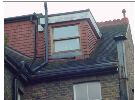
Rear dormer fascia requiring redecoration, due to their being no gutter. Also showing vent, please see item 2 below.
