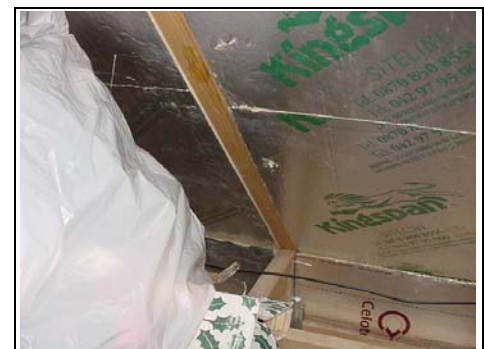
This photo shows the common rafters (the ones that form the pitch of the roof)
