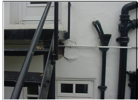
Cracking near rear fire escape.
