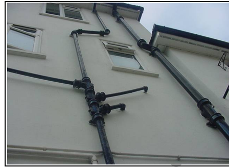
Cast iron soil and vent pipe
