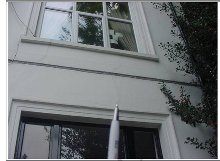
Crack around window Pen identifies the line of cracking.
