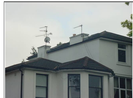
From this photo you can see the main roof is at various different
