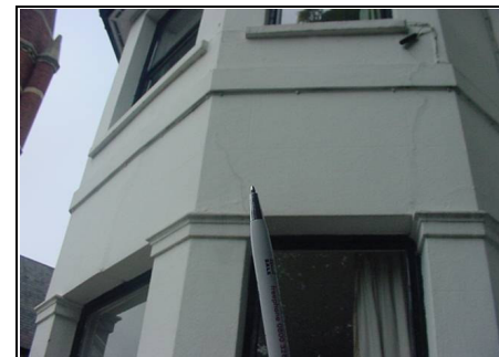
Crack above bay window
