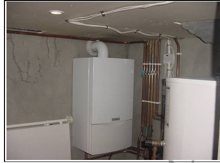
Boiler in basement
