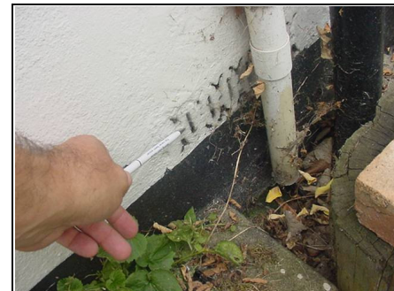
Partially blocked air brick
