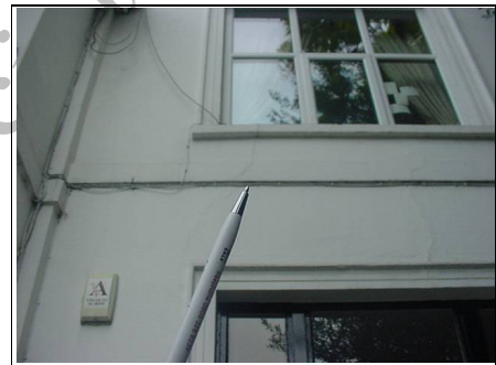
Crack above window
