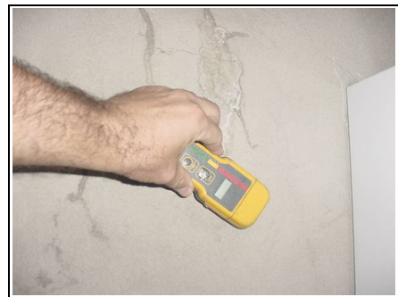
Dampness coming through tanking
