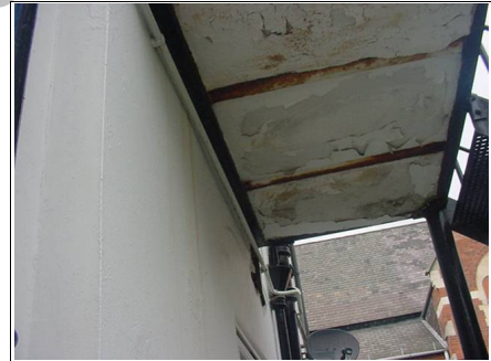
Rust on fire escape
