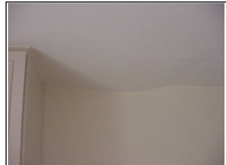
Dip in master bedroom ceiling
