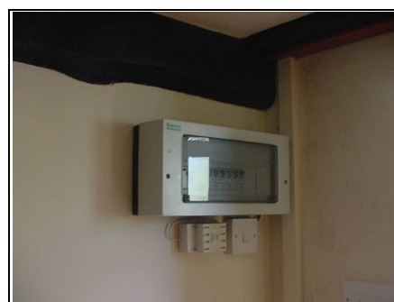
Electrics in annex
