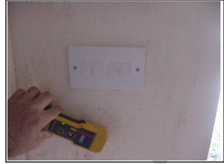
Finding lateral dampness
