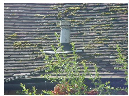
Plastic soil and vent pipe just visible to rear of property
