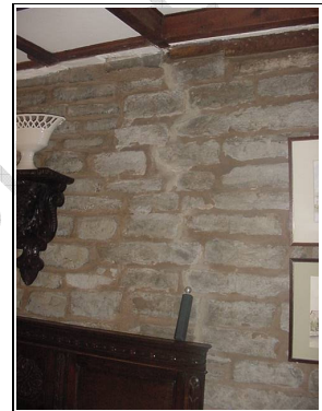
Cracking visible internally
