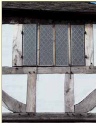
88A Church Street Tewkesbury: wrought iron casement & stay
