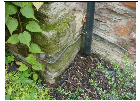
Water discharging against the property
