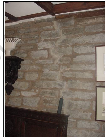
Crack internally in left hand wall
