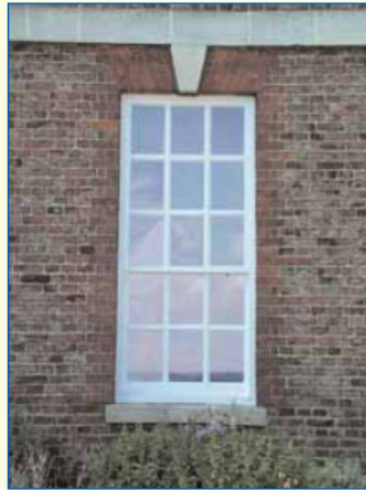
Wallsworth Hall Twigworth: mid 18th Century ovolo moulded sash window with rubbed brick lintel, stone cill and keystone
