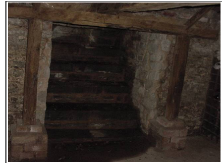
Dampness coming in through cellar flaps
