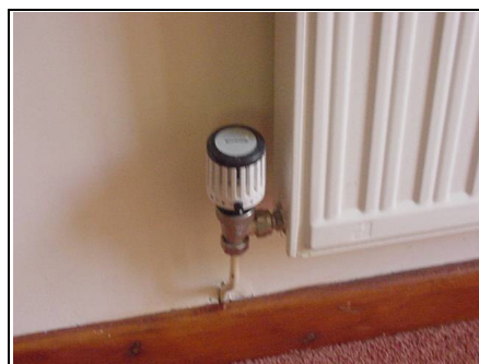
Microbore plumbing in annex
