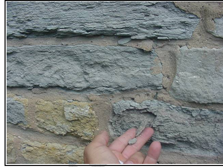
Close up of stonework deteriorating with face coming away
