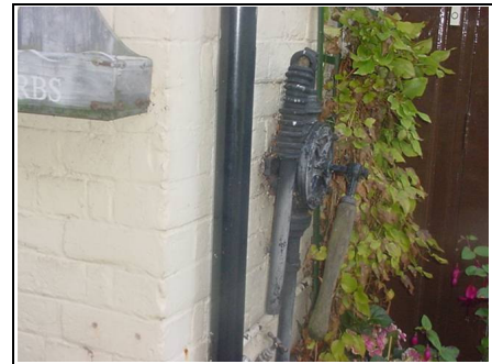
Electric pump from well (although old pump remains)
