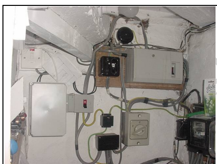
Electrics and generator switch
