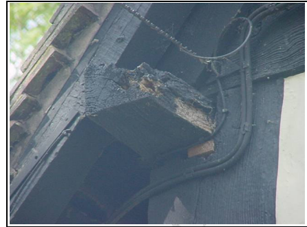
Active woodworm visible to purlins
