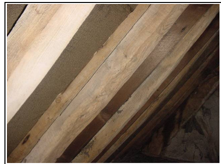
Some of the timbers have had new timbers put back to back, known as back to backing, to add strength
