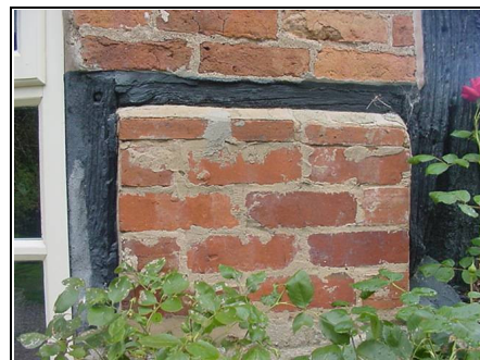
Poor cement mortar repairs to brickwork
