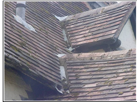
Valley gutters leaking
