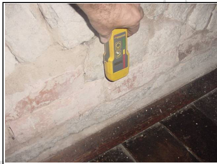
Finding rising damp
