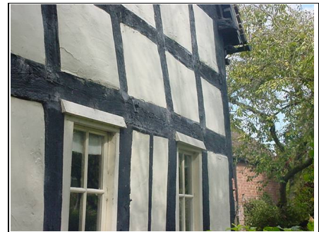
Bowing in right hand gable
