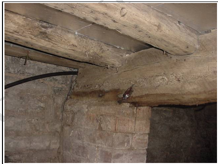
Dampness in timber – knife test into damp spine beam
