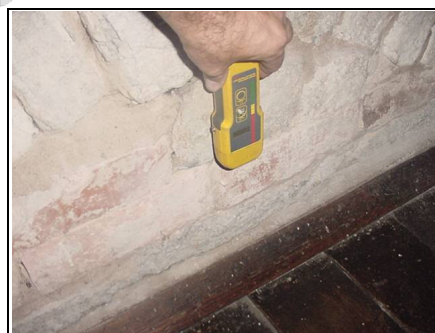
Finding rising damp
