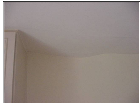
Dip in ceiling in master bedroom
