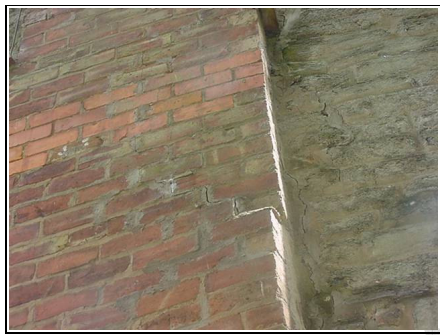
Cracking around left hand chimney
