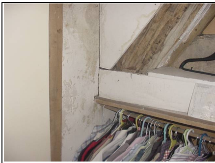
Dampness coming in from main roof
