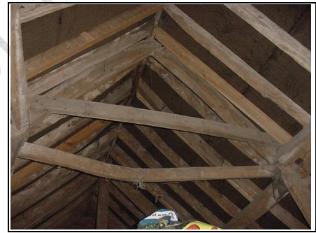
Broken collar truss in roof
