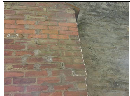
Crack in left hand chimney
