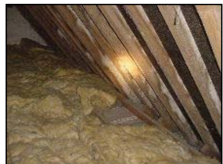
Note the white staining, which is condensation.
