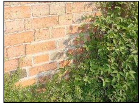
Structural movement to the front right hand corner.
