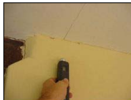
Hairline cracking between the plasterboard – fairly typical.
