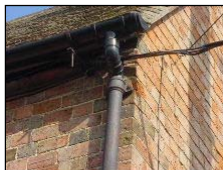
A close up of the plastic gutter leading into a cast iron downpipe.
