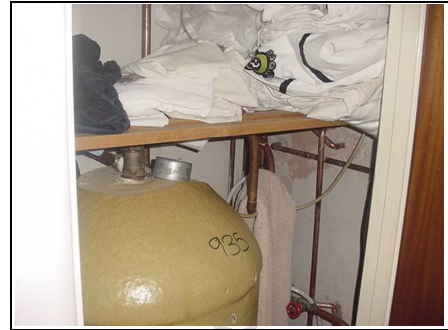
Hot water cylinder
