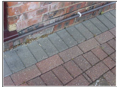
External gas pipes
