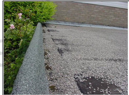
Leaking rear gutter
