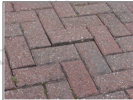
Front Garden – pavier lifting indicating some movement
