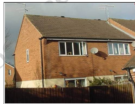
1980's property, cold bridging was found in the lintels
