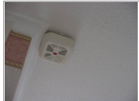
Battery operation smoke alarm
