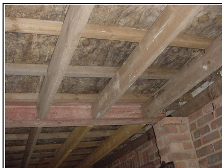
View inside garage roof, mould to the roof decking.
