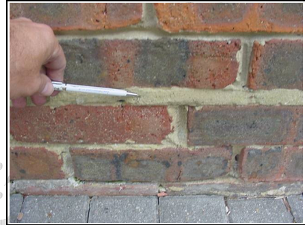
Main property damp proof course
