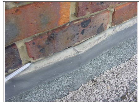
Flashing coming away to the right hand side
