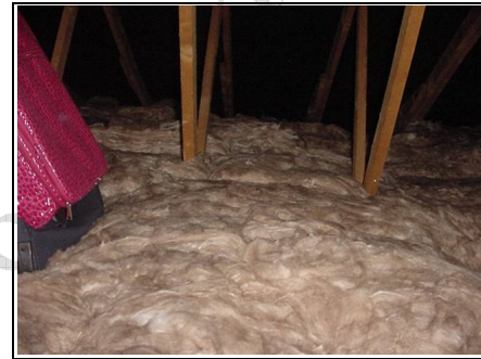
Roof space mass of insulation more ventilation required
