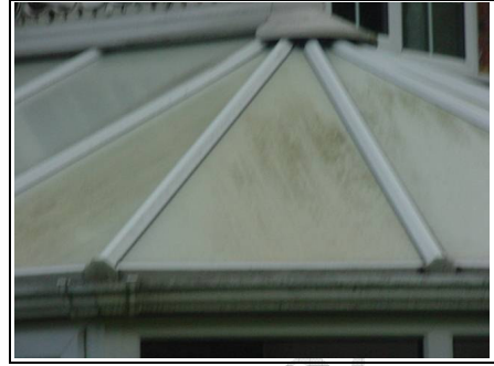
Moss starting to occur on conservatory roof
