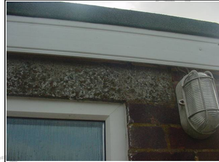
A close up view showing there is a concrete lintel over the door and window. This is where the cold bridging occurs causing condensation inside.
