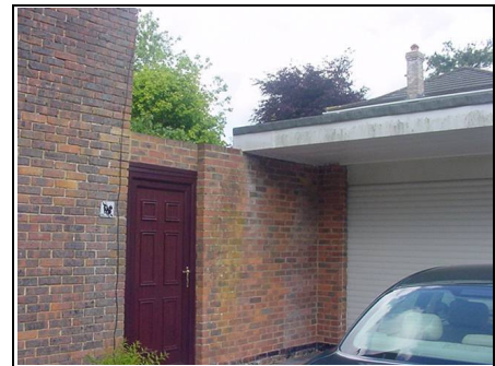
Moss to garage fascias and soffits
