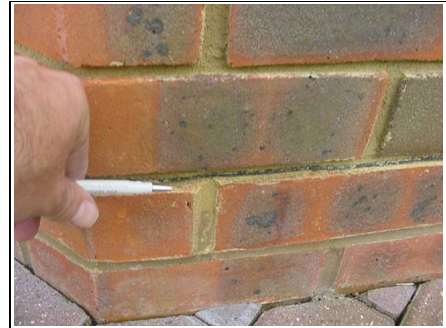
Kitchen/conservatory damp proof course
