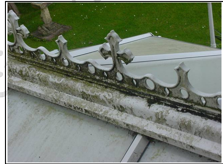
Mould to conservatory roof
