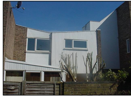
1970's property with cold bridging to the roof beams and the lintels
