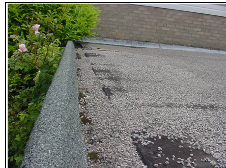
Rear leaking gutter to tree end
