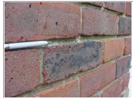
Close up of messy pointing to brickwork
