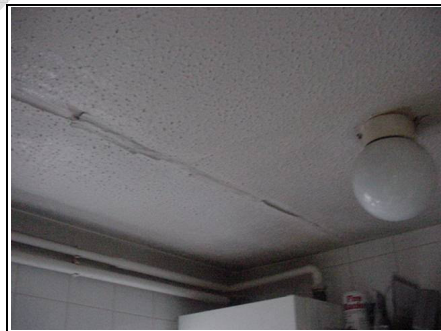
Leak in utility room
