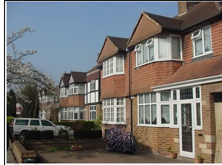
Post war / 1950's property that cold bridging can be a problem in.
