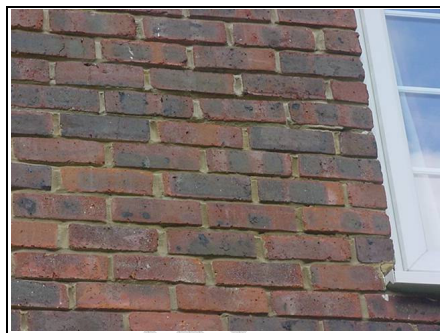
Messy pointing to brickwork
