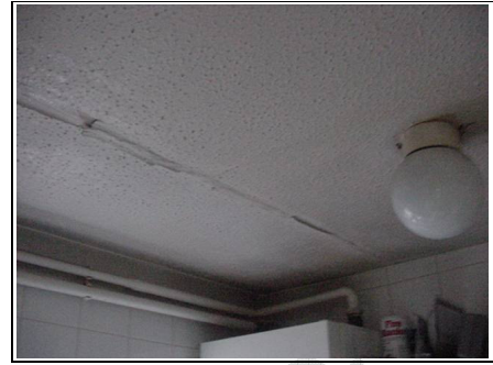
Leak in utility room
