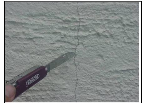
Hairline cracking to left hand side of property which runs all the way
