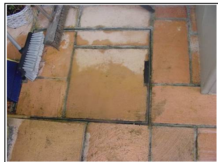
Manhole, near conservatory
