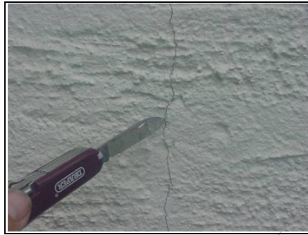
Hairline crack left hand side — marked by the penknife
