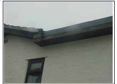
Minor deterioration to fascia board to the flat roof area
