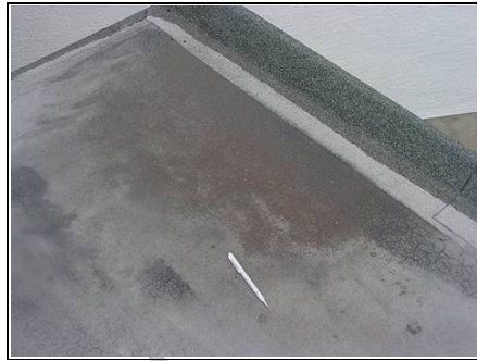
Ponding on flat roof
