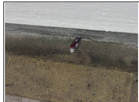
Cracking on left hand side of balcony
