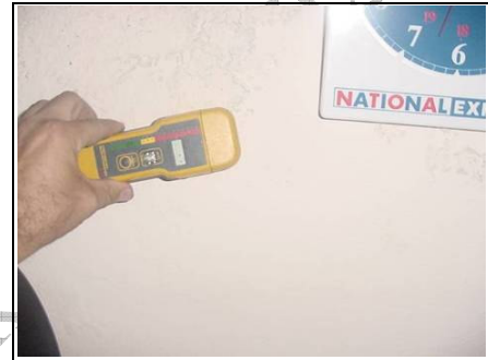
Finding lateral dampness coming through rear wall
