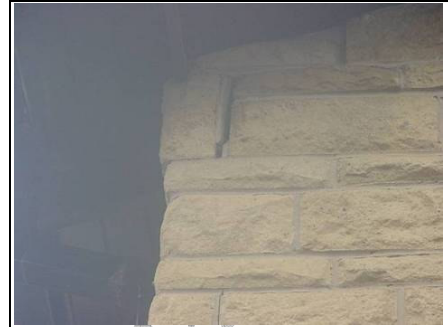
Stone work coming away
