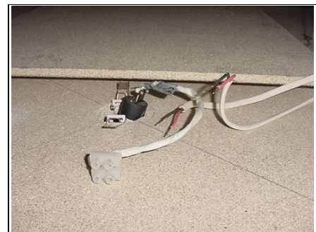
DIY electrics –cable connector hard core undone
