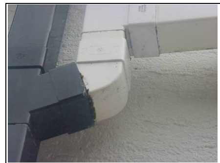
Leaking downpipe from conservatory roof
