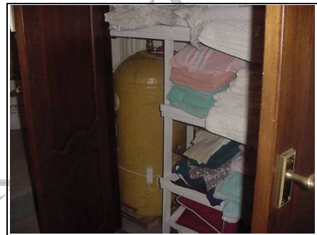
Factory insulated cylinder
