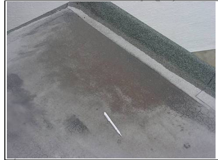
Ponding to the roof
