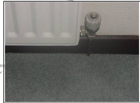
Microbore pipe system
