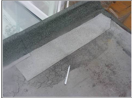
Old patch repair and crocodiling
