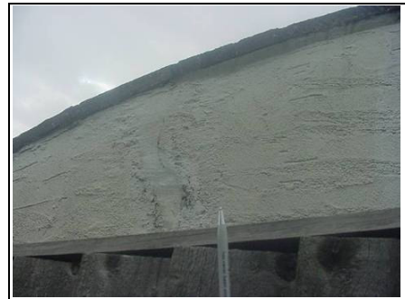
Movement visible to right hand side
