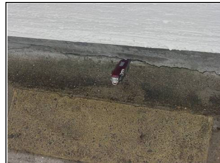
Cracking to balcony areas that need to be re-masticed
