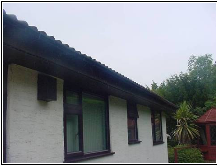
Cracks to blockwork of the property
