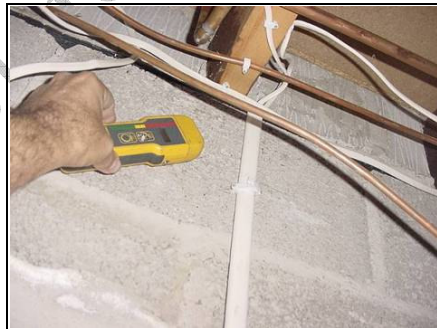
Checking for dampness on ceiling in bar area
