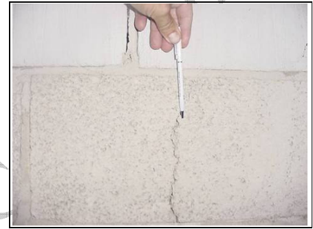
Crack to gable end on right hand side, taken within roof space. We also noted there was a different type of brick from the top to the bottom
