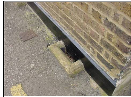
The edging around the airbrick stops rain water getting in
