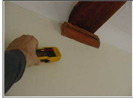
Looking for lateral damp
