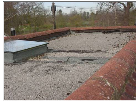
High Level Flat Roof Awkward central drainage valley
