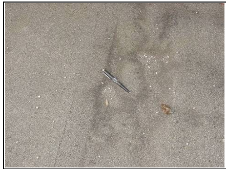
Close up of the blistering to the felt to the lower level rear flat roof.
