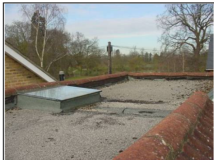
General View of high level flat roof. The roof window in this photo is the one that gives light to the shower room.
