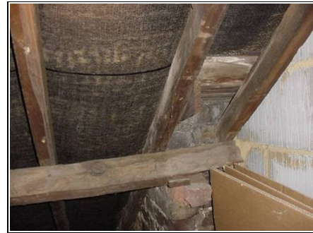
Close up of the purlin to the front of the property that needs a prop.
