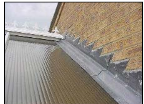
The polycarbonate conservatory roof meeting the main building with a lead flashing.
