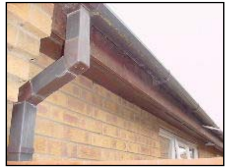
Minor leaks to the downpipes
