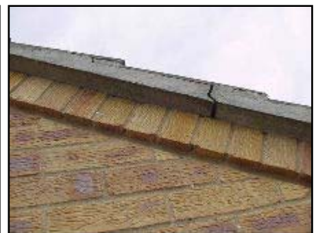
Splitting to the gable perimeter concrete, this needs sealing.
