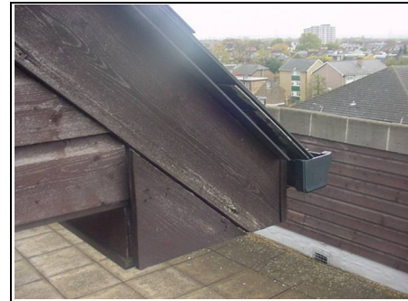
Verge where cement has come out
