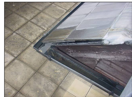
Verge showing signs of dampness getting in
