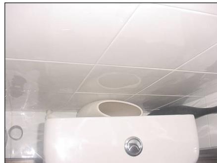
WC cistern not supported
