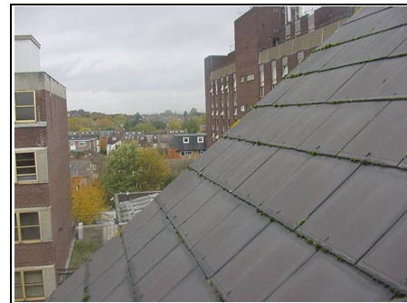
Moss on man-made slate tiles
