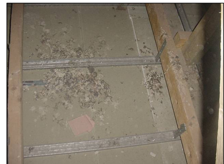
We noticed pigeon droppings in the roof
