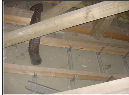
Extractor fan not extracting to outside air
