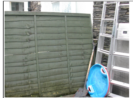
Timber fence in poor condition
