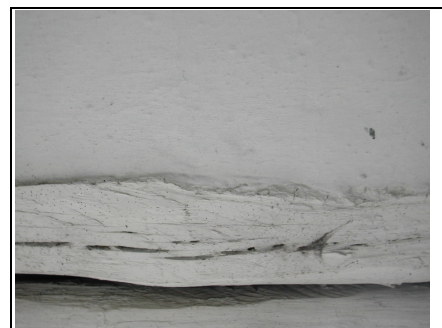
Signs of woodworm activity in timber in roof above passageway
