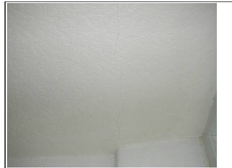
Hairline cracks to ceiling
