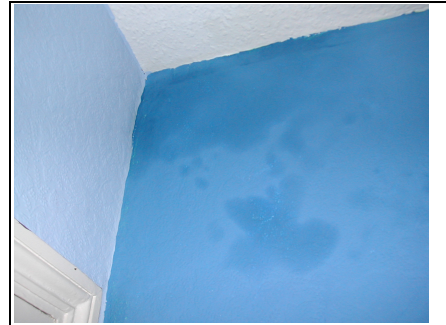
Damp ceilings and walls
