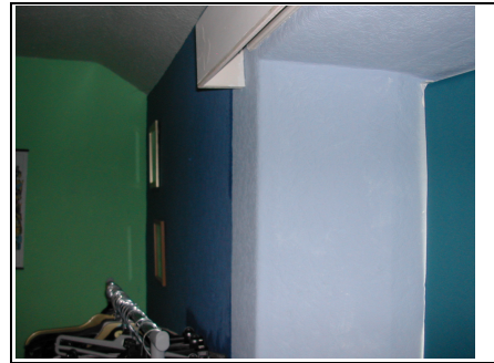
Wall appearing to bow
