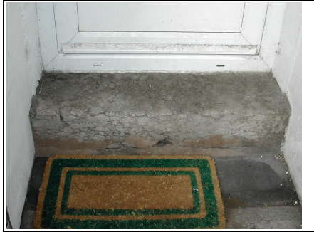
Front door and cracked door step
