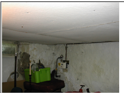
Excessive damp in cellar
