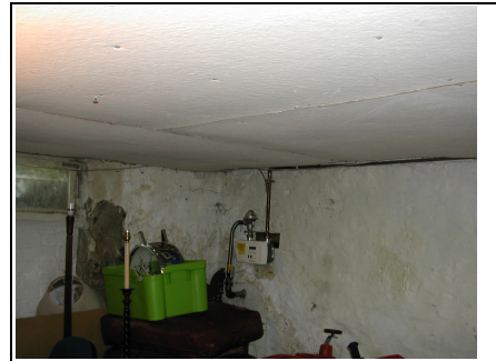
Dampness in cellar
