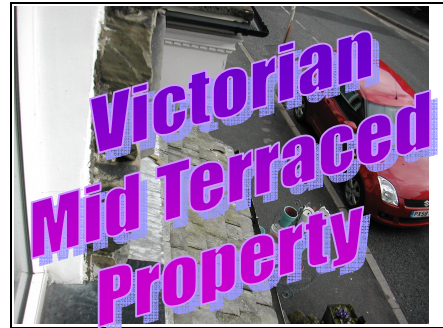
Slipped slates on porch
