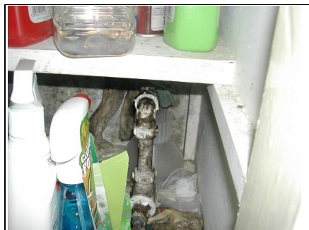
Stopcock under kitchen sink
