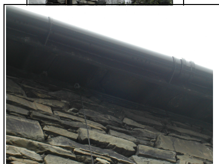
Plastic gutter to rear
