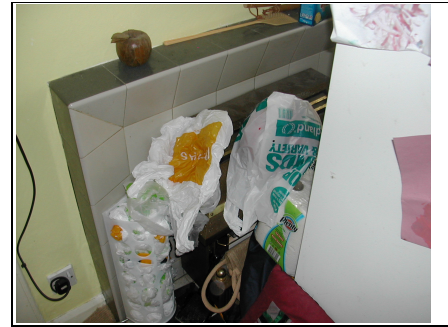
Kitchen gas fire
