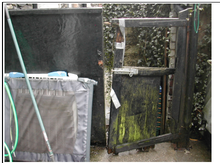
Dilapidated gate to courtyard
