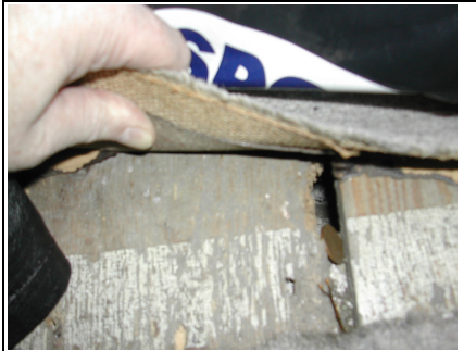
Evidence of woodworm in front bedroom
