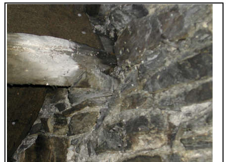
Purlin requiring repair
