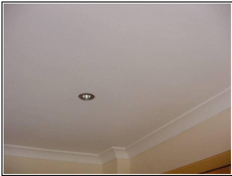
Ceiling light in the kitchen
