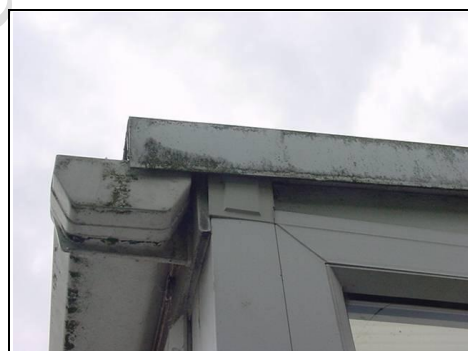
Discoloured plastic on conservatory needs cleaning
