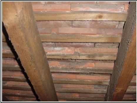
Back of the tiles, some have been replaced and some are spalling.
