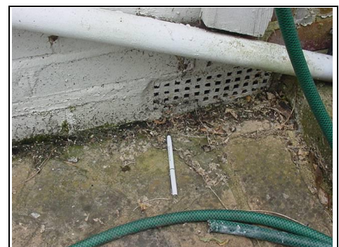
Air brick acting as a gutter
