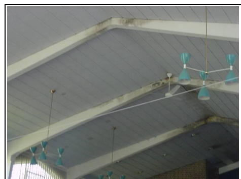
Cold Bridging in a commercial property with a concrete frame.
