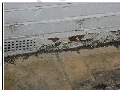
Water damage at base of property
