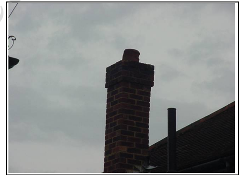
Left chimney is leaning over
