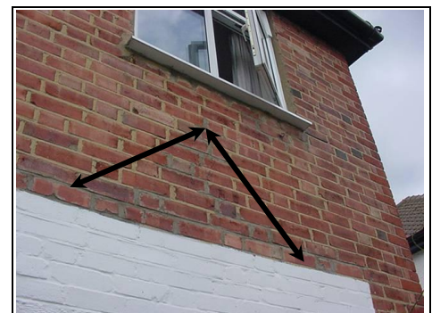
Different coloured mortar in an 'A' shaped pattern below the window indicates there has been movement
