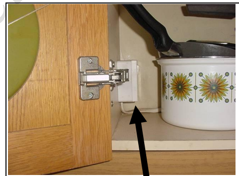
Socket point in the cupboard
