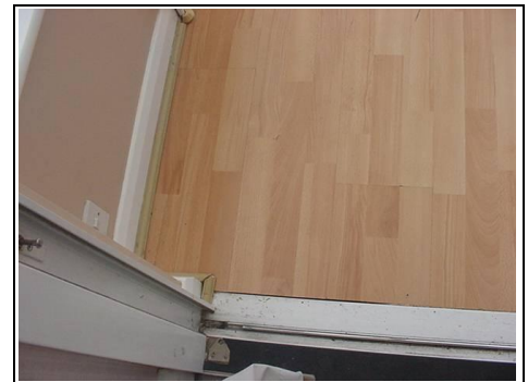
Poor quality laminate flooring with quadrant bead.
