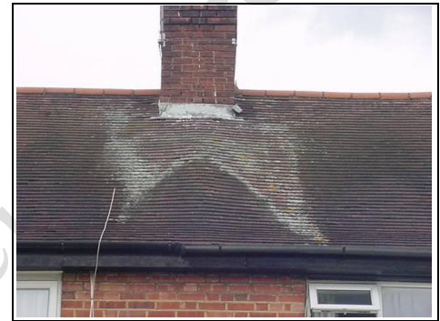
Dip in the main roof to the rear
