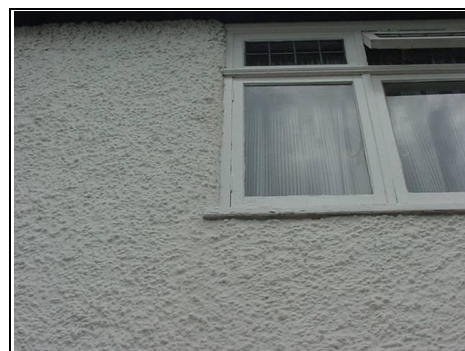
Some windows did not have sills
