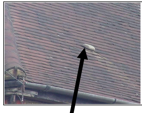
A close up of this roof shows a mushroom vent indicating a new roof probably from the 1980's
