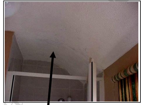
Dampness above shower (sorry this is not very clear in the photo)
