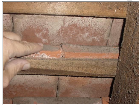
Closer still this shows dampness coming through
