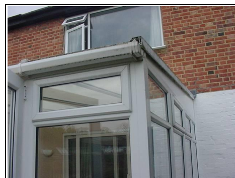
Conservatory does not have trickle vents
