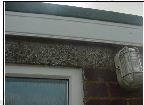
A close up view showing there is a concrete lintel over the door and window. This is where the cold bridging occurs causing condensation inside.
