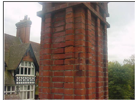
Weathering to chimney
