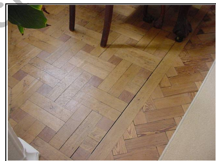
Flooring blocks covering the floor were opening up slightly
