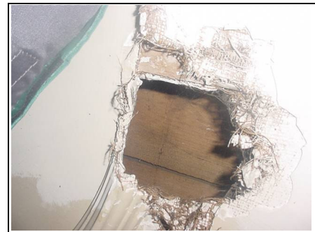
Small hole in lining with close boarding behind it
