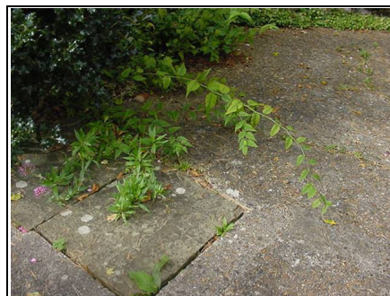
Manhole not lifted
