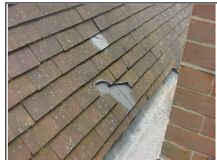
Poor repairs to roof tiles
