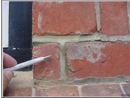
Poor repairs carried out to cement mortar
