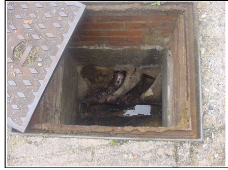
Drain at front with tree roots in it
