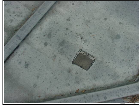
Poor repair to lead
