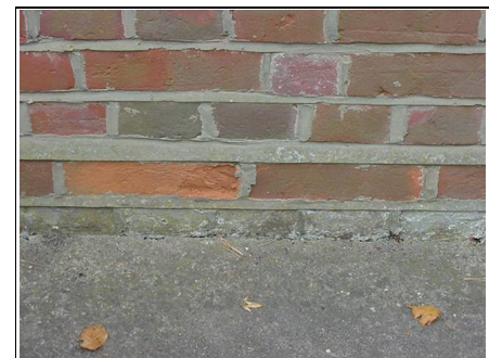
Cement causing spalling to the brickwork makes it more vulnerable to dampness
