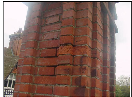
Close up of chimney that needs re-pointing
