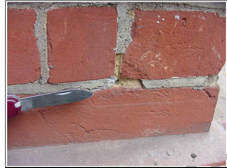
Cement mortar coming away to reveal original lime beneath
