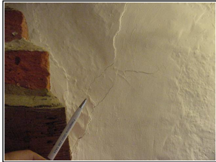
Cracks to right hand chimney
