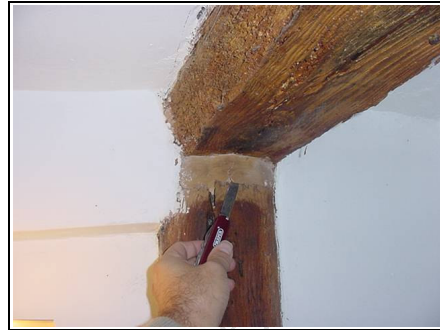
Spine beam and floor joist – filler in timber supports indicates previous repairs
