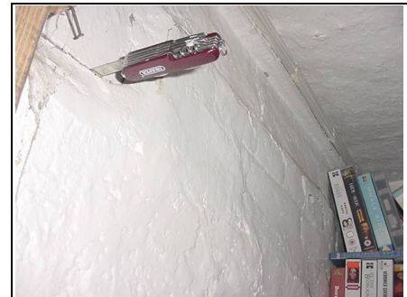
Cracking to right hand side of breast of beam in adjacent cupboard
