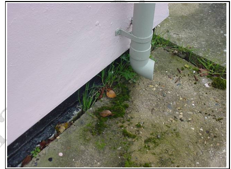
Water logging to rear left hand side allowing grass to grow
