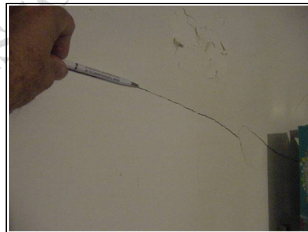
Cracking in utilities room
