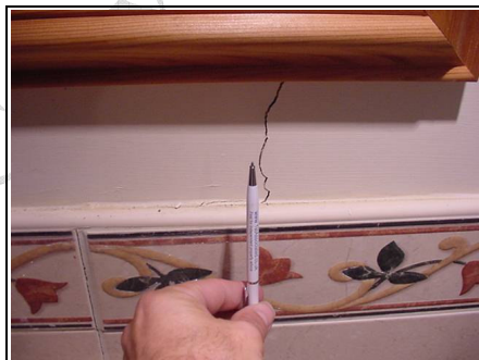
Cracking to bathroom
