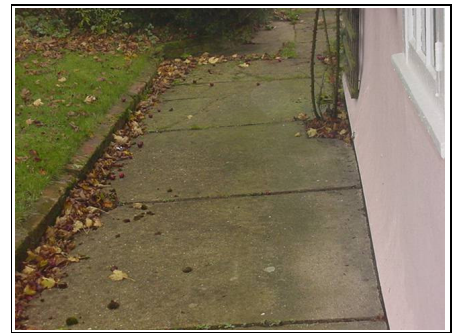
Concrete slabs around prop that indicate that major work has been carried out to foundations
