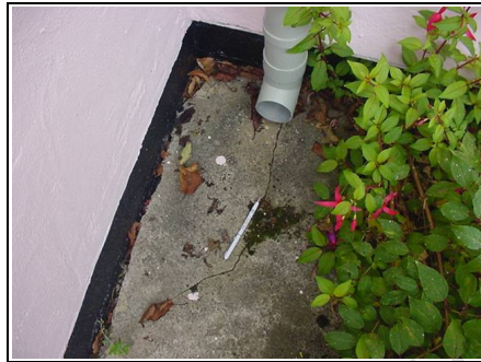
Cracking to ground near bathroom
