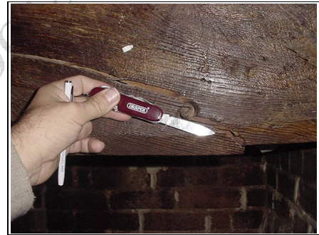
Cracking to chimney breast beam
