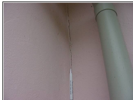
Cracking to bathroom
