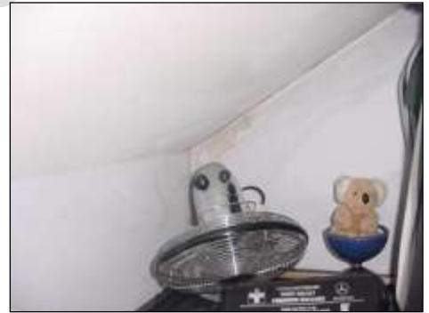
Dampness within top bedroom front left hand corner
