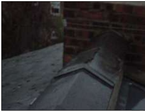
Damaged coping stone that has been put back
