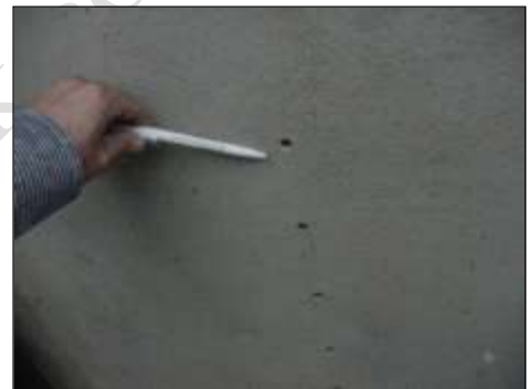
Wall showing holes where DPC has been inserted
