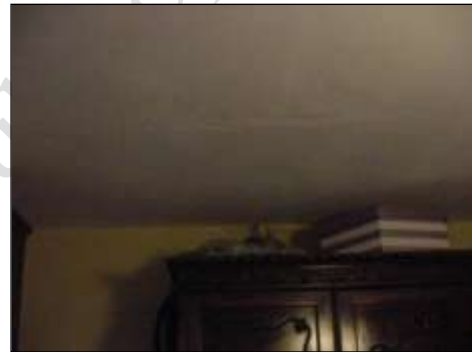
Dampness within main bedroom left hand wall
