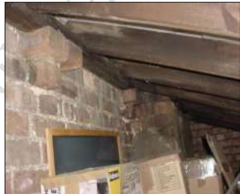
This is where the parapet wall starts to the left hand side of this photo
