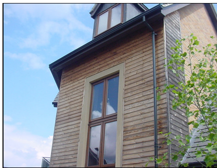
Pattern staining that can occur to untreated cladding
