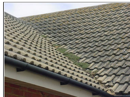
Valley gutter needs cleaning.
