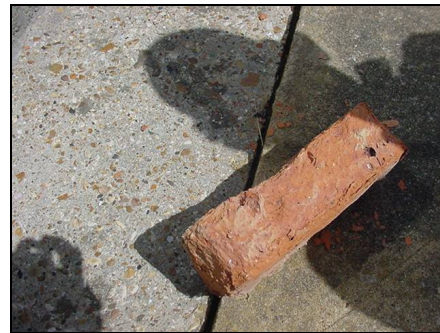
Deterioration to rear of brickwork
