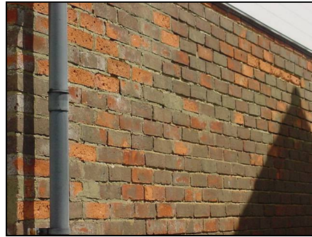
Poorly repointed brickwork
