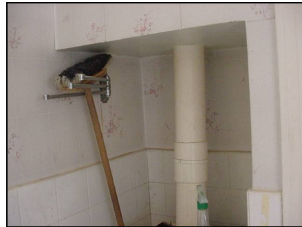
Vent coming from the boiler system
