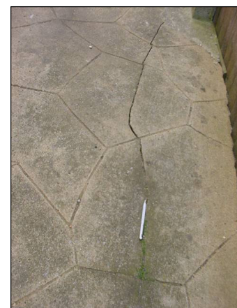
Cracking adjacent to drains
