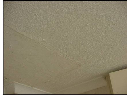
Possible asbestos to ceiling paint commonly known as Artex
