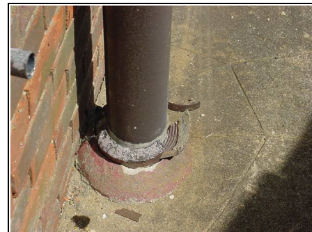
Soil and vent pipe
