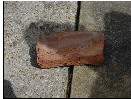
This brick shows spalling to front and rear
