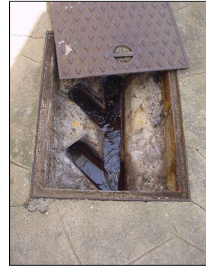
Drain lifted close to entrance door
