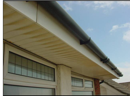
Fascia board in need of attention
