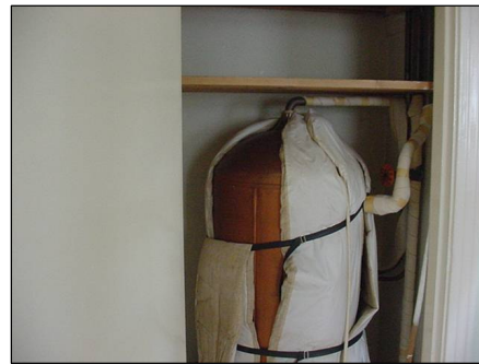
Old hot water cylinder
