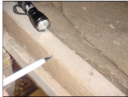
Woodworm in the roof
