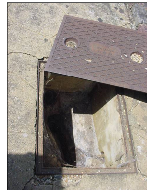
Drain lifted front corner
