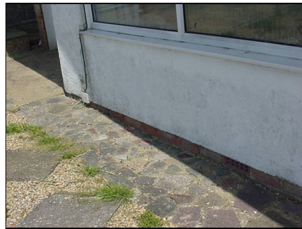
Area needs a French drain front left hand corner
