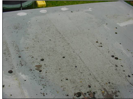
Ponding on roof
