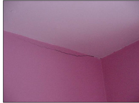
Crack to WC wall
