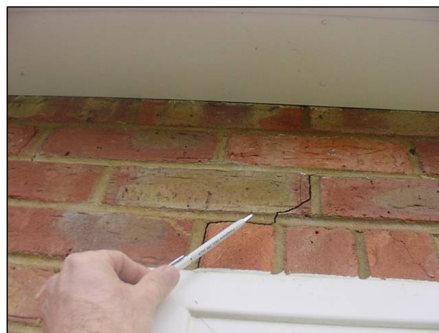
Cracking on neighbours side
