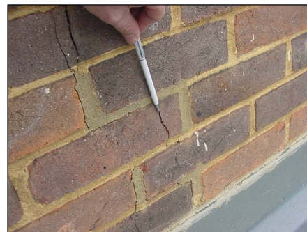
Cracking in rear wall (old main wall of property)
