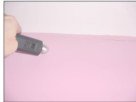
Taking damp meter reading on cracked WC wall - 21
