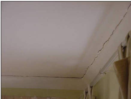
Cracking to the ceiling
