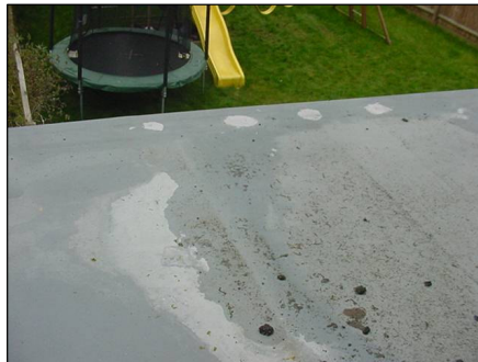
Ponding on the roof
