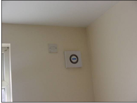
Extract fan requires independent operation in bathroom
