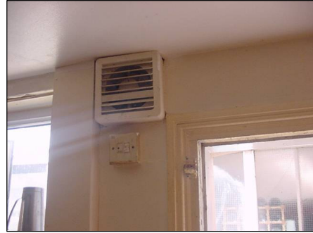
Extract fan within the kitchen has to be independently operated and was working at the time of the report
