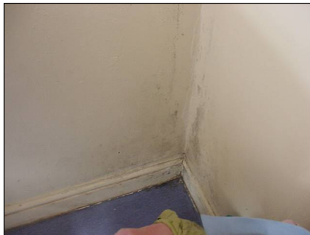
Damp in front right hand corner of bathroom
