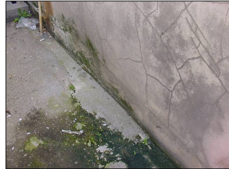
Hairline cracks to render to rear of the property needs to be redecorated and sealed
