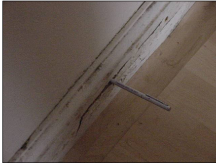
Possible wet rot to the skirting between the front lounge area and the rear kitchen/bathroom needs further investigation
