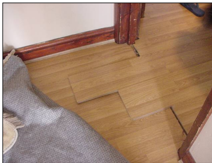
Flooring not secured
