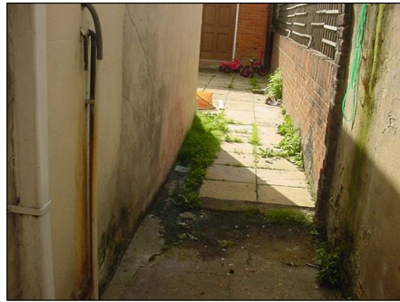
Water sitting against property due to the high level of ground requires a French gully
