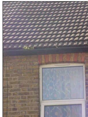
Gutters require cleaning
