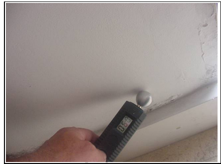
Damp meter reading of 90 in kitchen
