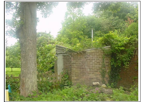
Shed with dilapidated roof
