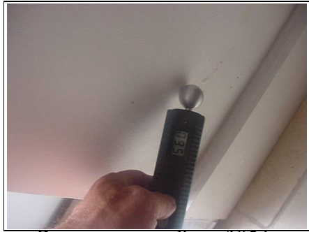
Damp meter reading of 95 in kitchen
