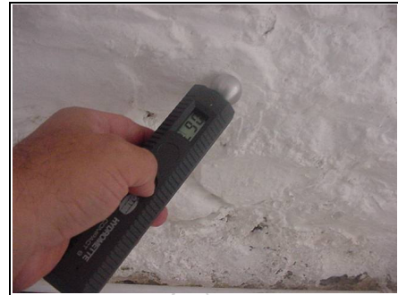
Damp meter reading of 67 to shower room
