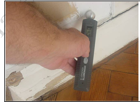
Damp reading of 40 to rear reception room
