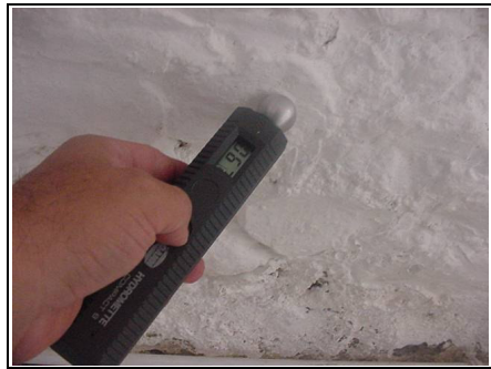
Damp meter reading of 93 to shower room
