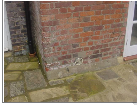
Rustic paving slabs – ground level needs lowering
