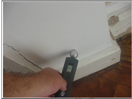
Damp reading of 63 to rear reception room
