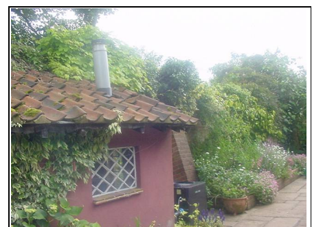
Swimming pool outbuilding (with buttress just behind it) which has been in place for 30
