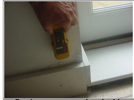
Protimeter was used to double check meter readings
