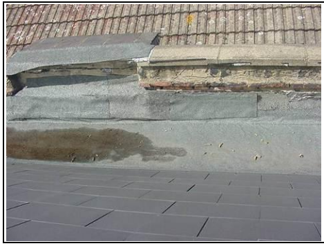
Lack of any decent flashing at all to the middle and front of the right hand valley gutter
