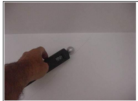
Hairline crack with reading of 28
