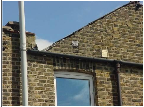
Gable end showing that there should be mortar or an end cap to the roof
