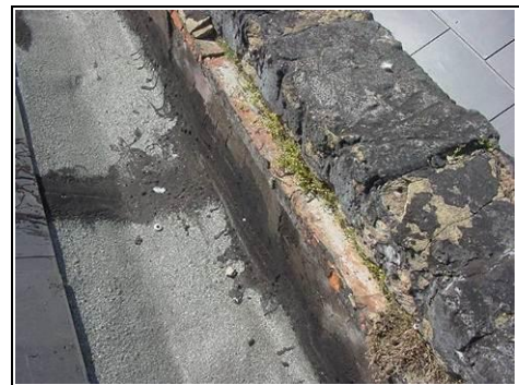
Bitumen repair. Also note the parapet wall is letting in water which is why the plants are growing from it
