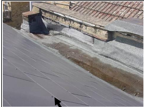
How the slates should be fixed with a nail(or tingle) as they are to the front.
