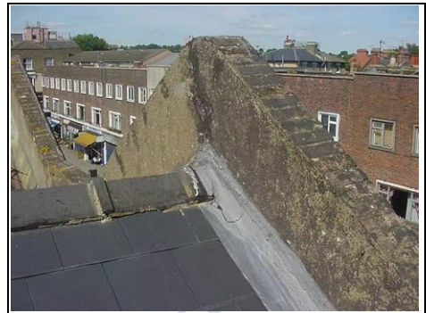
The felt does not lap underneath the slates correctly. We would expect this to lap by at least two slates which is typically half a metre. In this case it is barely 100mm.
