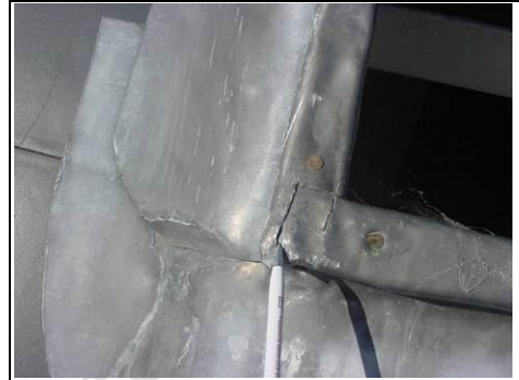
Damage to the lead
