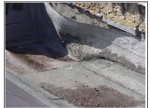
Felt flashing that is coming away. Lead should have been used.
