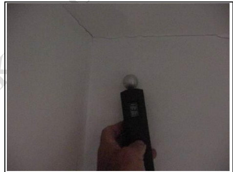
Reading of 33 on the Gann meter. This is acceptable but the hairline cracking does suggest something has occurred
