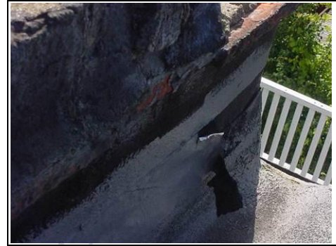
Flashband repairs to the rear of the left hand valley gutter have come away
