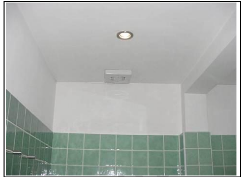
No problems at high level
