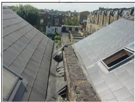
Many slates have been damaged
