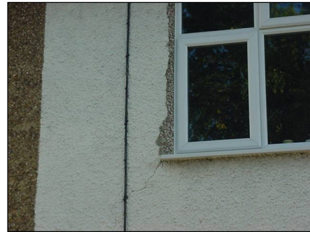
Cracking to the lower right hand corner of the rear right hand window
