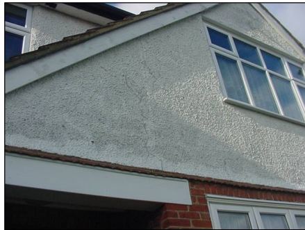
Cracking to render at the front of the property where water will be getting in
