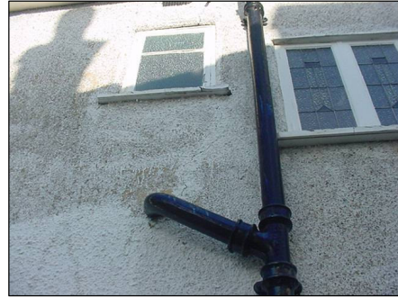
Cast Iron soil and vent pipe
