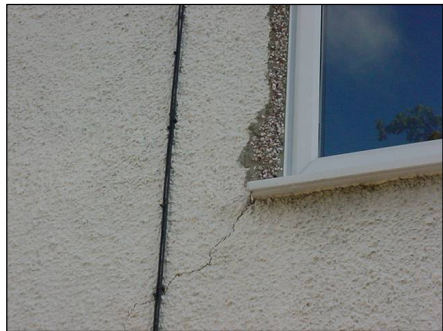
Cracking to render at the rear of the property to the corner of the plastic window
