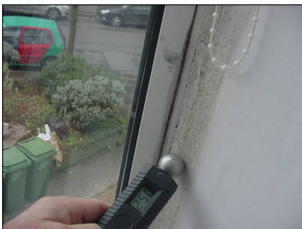
Mould and damp reading next to window front bedroom
