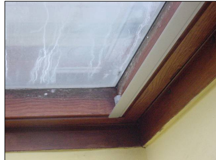
Condensation to top floor loft conversion bedroom window
