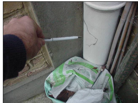
Cracking to cast iron downpipe
