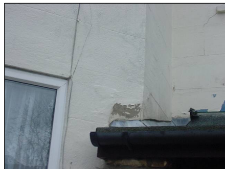
Hairline cracking around window to entrance area
