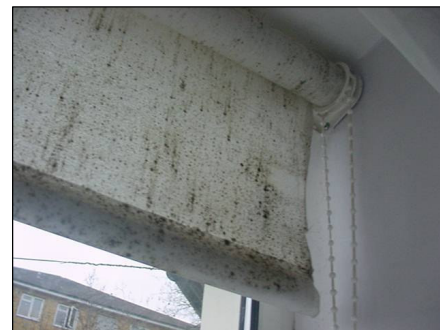
Mould on blind in front first floor bedroom
