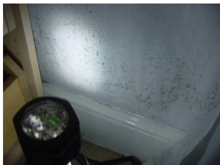
Mould adjacent to cupboard first floor bedroom
