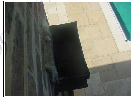
Junction detail to the hopper head not finished correctly
