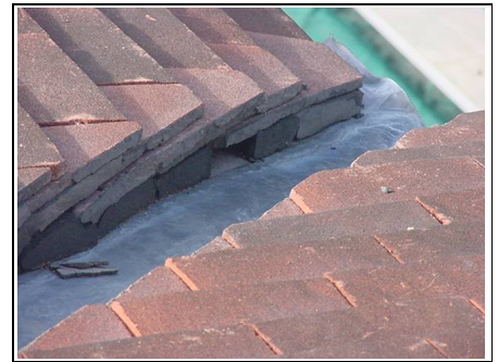
Valley gutter starting to deteriorate
