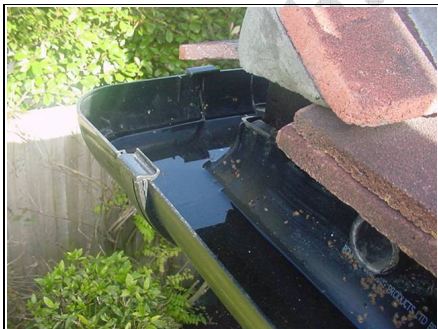
Gutters not clearing rainwater rear right hand corner, the fall also needs to be checked
