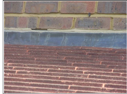
Poor flashing detail not only is the flashing not high enough it has also not been bedded correctly. The cement fillet has come away from the lead flashing.
