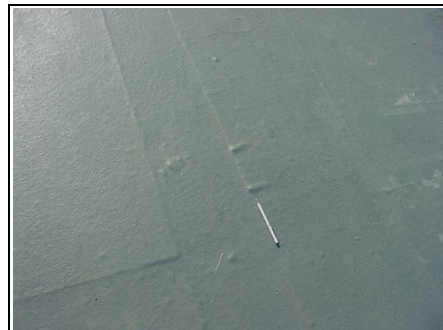
Blistering in the flat roof
