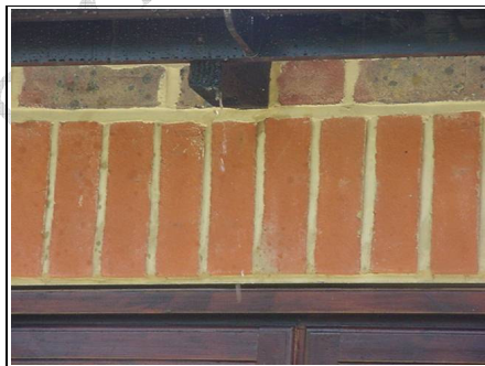
Water missing the gutters and coming down the wall
