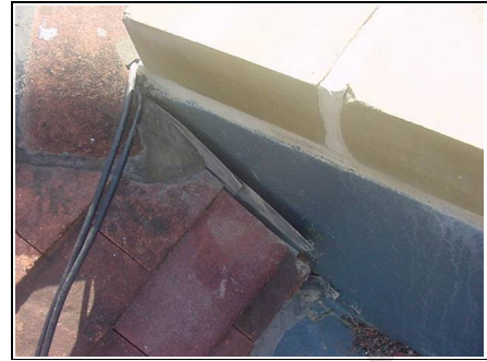
Poor lead gutter detail
