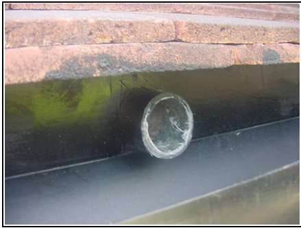
Poor gutter detailing
