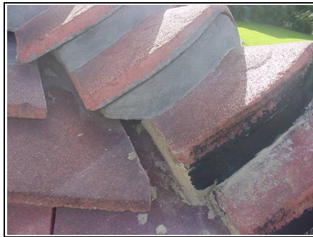
Poor ridge tiles detailing
