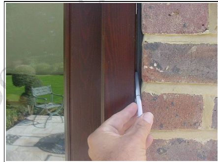
Mastic not applied
