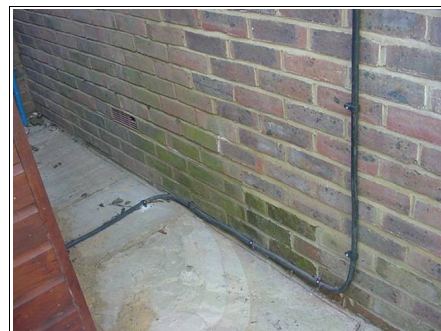
Result of overflowing
