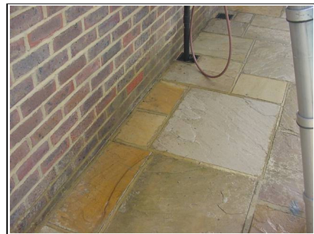
Water missing the gutters and coming down the walls
