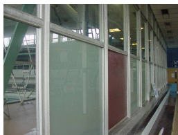
Degrading metal frame to curtain walling
