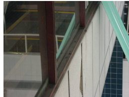
Damage and deterioration to ceiling tiles
