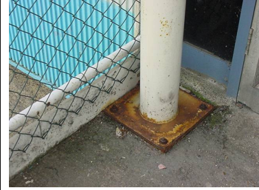
Corrosion to base of entrance canopy
