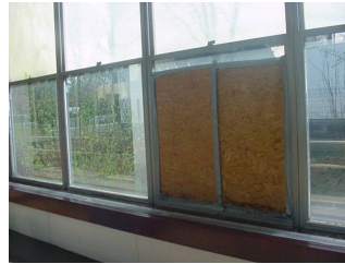
Broken rear window
