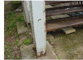
Rusting steps and staircase structure
