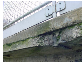
Deterioration to ramp
