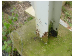
Rusting to base of stairs
