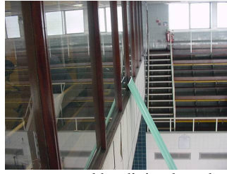
Damage caused by diving board
