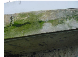
Moss and deterioration
