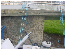
Crack in ramp up to learners pool
