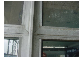
Close up degrading metal frame
