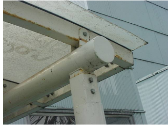
Corrosion to top of entrance canopy
