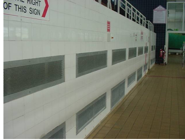
Corrosion to fixing screws around vents
