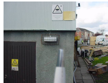
Hairline cracking right hand side
