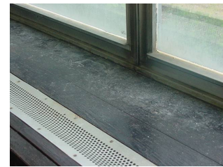
Damage to windowsill
